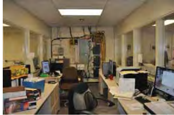
Figure 1C-83: Glazed service room between the two reprographic areas in Building 37.
