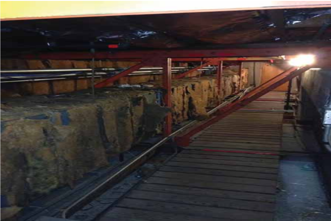
Photograph 2-General view of the suspect building materials, catwalk area
