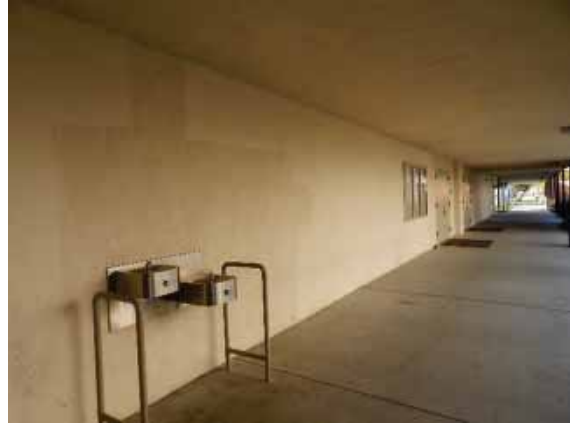
Figure 153: Visible patching of stucco on east façade of Music Building (Bldg. 2).
