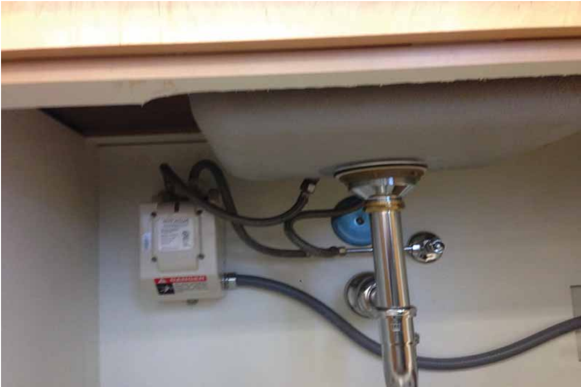
Photograph 7-View of the suspect asbestos under sink
