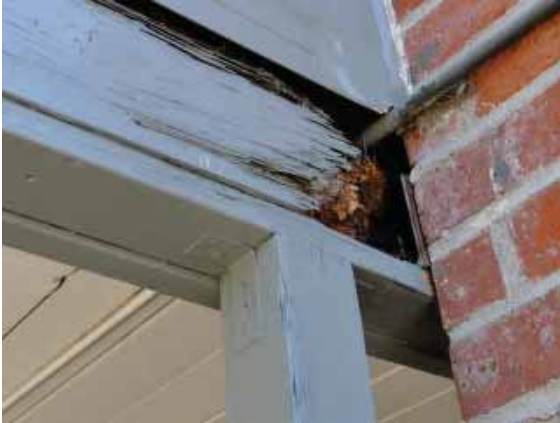
Figure 117: Wood decay in the walkway soffit at Building 9.
