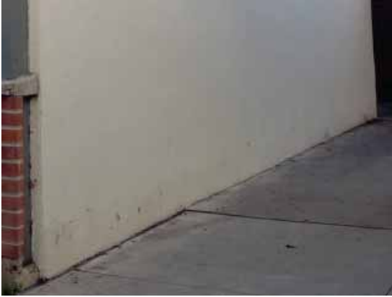
Figure 167: West façade of Building 36 with a low level of soiling and paint deterioration at base.
