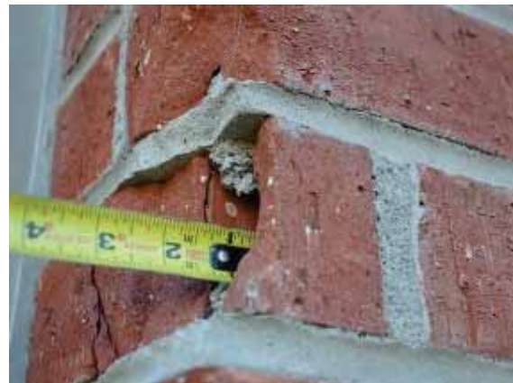
Figure 128: Heavily cracked brick with material loss at the northeast corner of Building 12.
