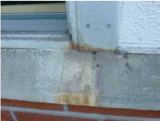
Figure 171: Rust staining at the window sill on the north façade of Building 36.
