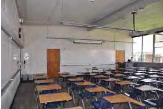
Figure 1C-74: Typical classroom in Building 35 and 36. Note the original internal doors and I beam and attached acoustical board tiles at the ceiling.
