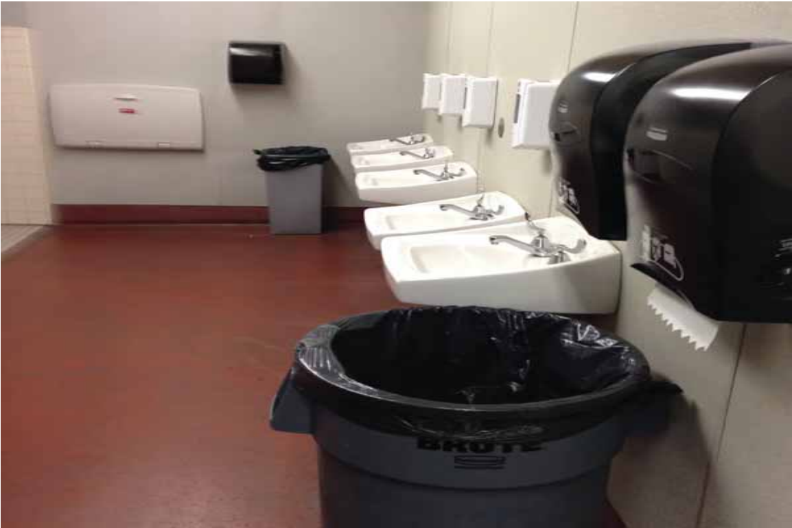
Photograph 7-View of suspect lead containing ceramic tiles, Toilet bowls, sinks and urinals in the restrooms
