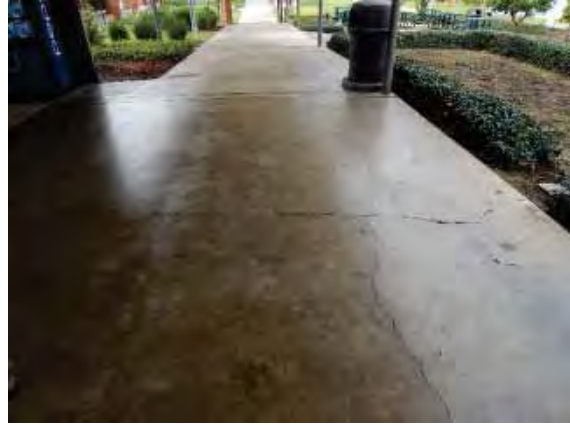
Figure 159: Cracking in the paving of the east-west walkway to the north of Building 2.
