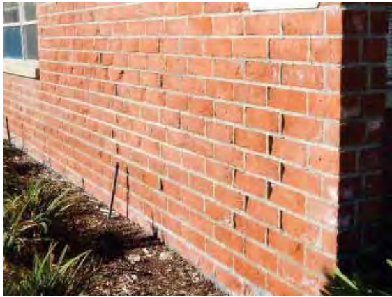
Figure 100: Spalling brickwork on the east façade of Building 8.
