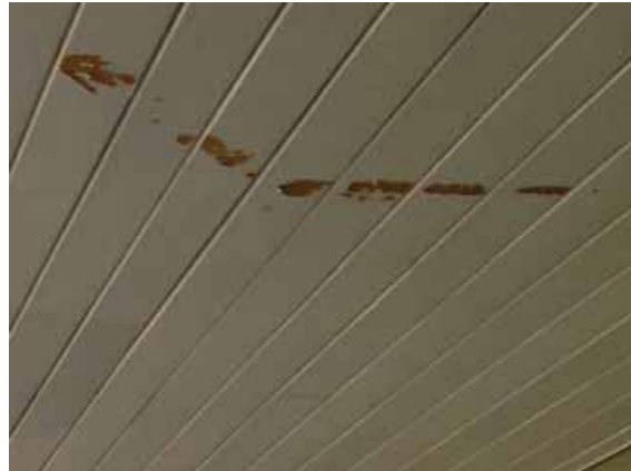
Figure 181: Scratched or peeled paintwork on the canopy roof at the west side of Building 37.
