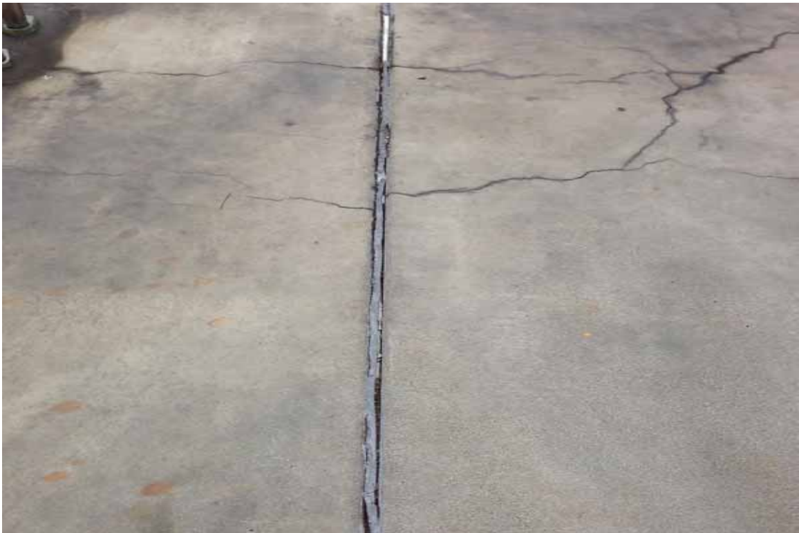
Photograph 3-View of the suspect expansion joint, building 93
