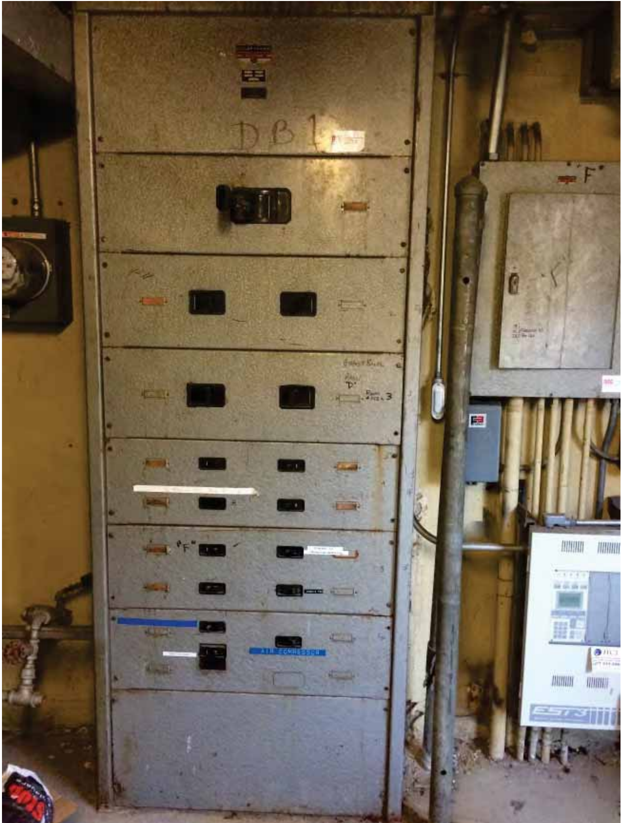
Existing distribution board DB1 and panelboard F original to building
