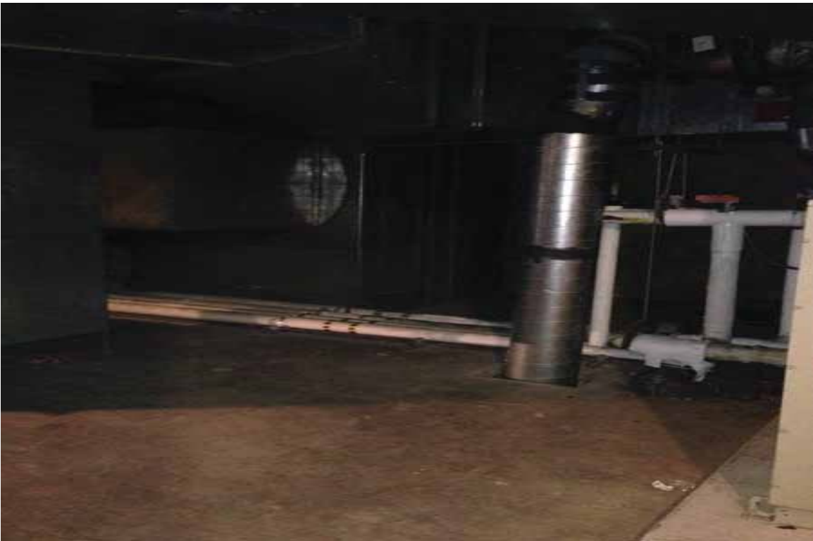
Photograph 3-General view of the suspect pipe insulation, plaster, drywall/joint compound, and HVAC mastic, mechanical room
