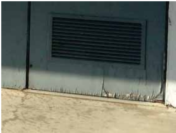
Figure 174: Water damage at the base of the door on the east façade of Building 35.
