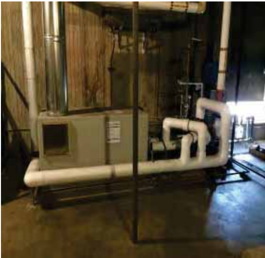
Lochinvar Boiler within Mezzaine
