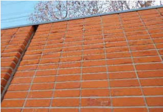
Figure 193: Around 50% of the bricks show some surface spalls.
