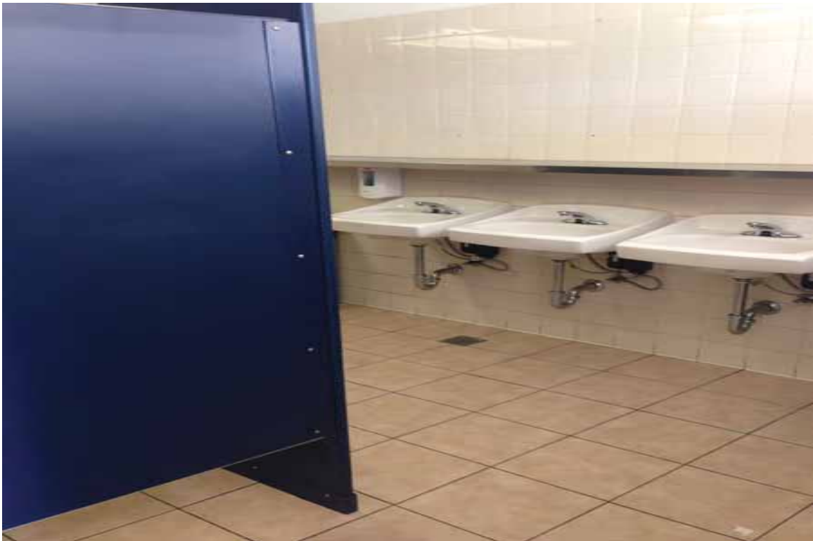
Photograph 11-Suspect lead containing ceramic tile & drain in the restrooms
