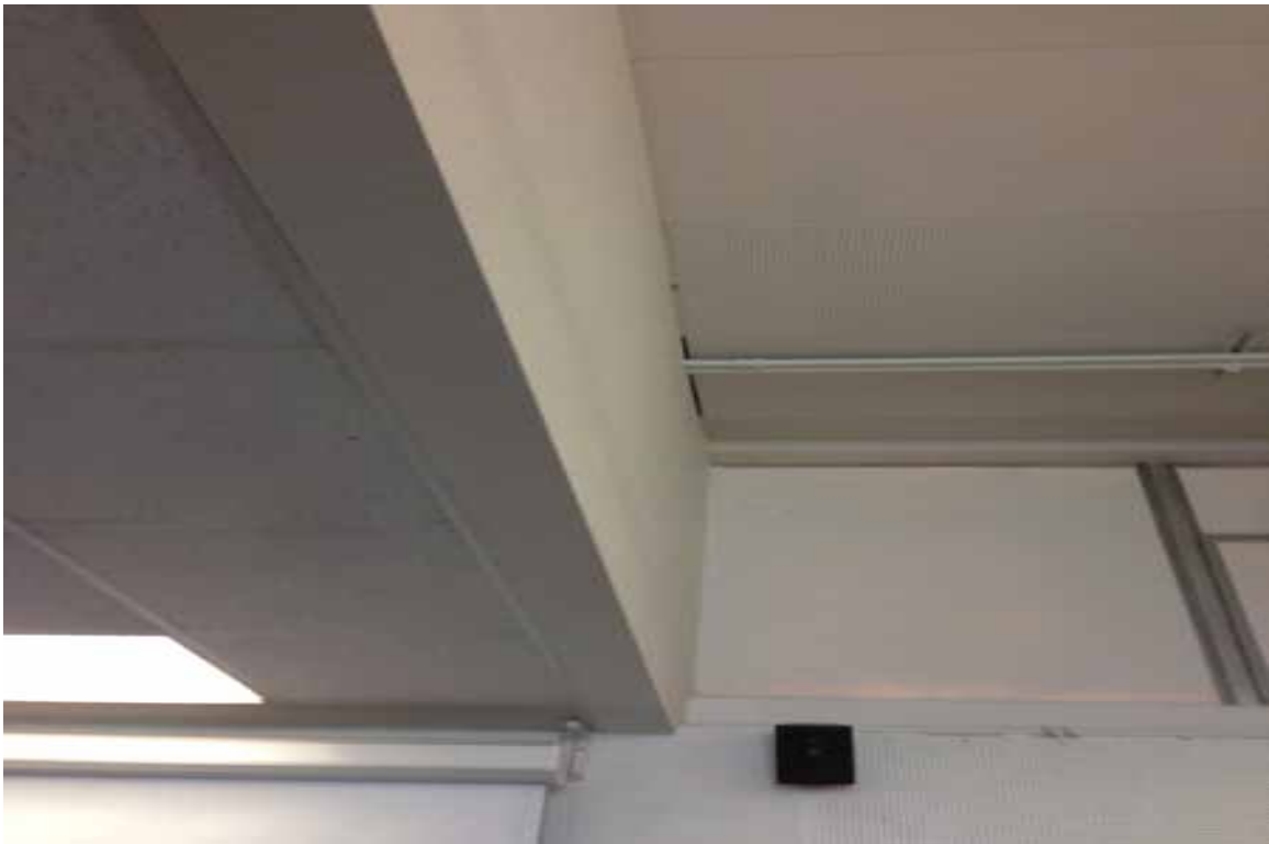
Photograph 9-General view of the suspect ceiling panels
