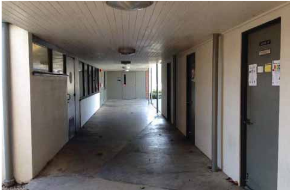
Figure 1C-85: Building 37's west façade along the covered walkway with door to the southeast classroom at the background. Building 38's east façade is at the right. The walkway with the tongue-and-groove ceiling is perpendicular of Building 35 and 36's south façade walkway.
