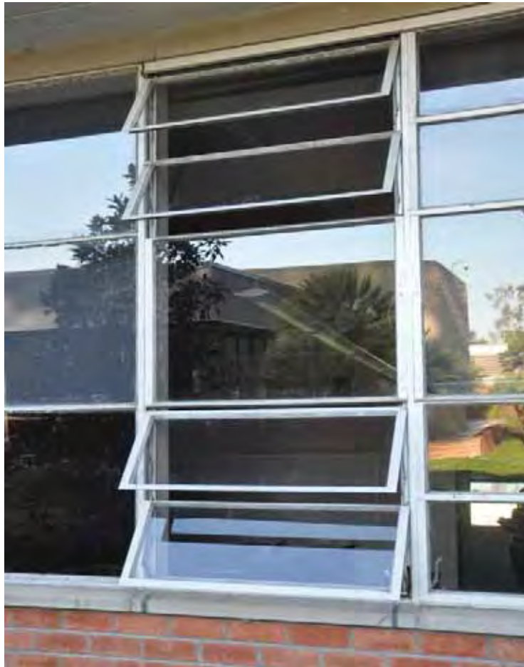
Figure 1C-36: Typical Building 12 and 13 windows with four awning windows connected and operated by one crank.
