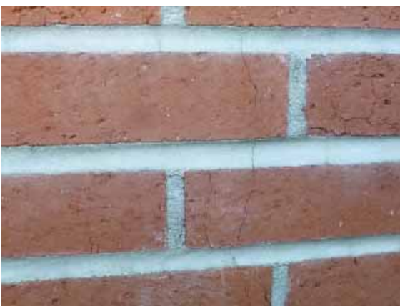
Figure 163: Hairline cracks on north façade of Building 36 on individual brick and running vertically up the wall through the bricks and mortar.
