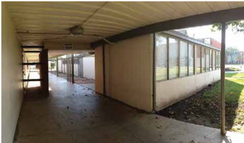
Figure 1C-84: View along Buildings 35 and 36's south covered walkway facing east with Buildings 38's stucco north façade and glazed west façade. Just visible in the background is the north façade of Building 37.
