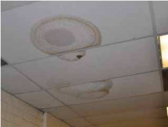
Figure 184: Water damage classroom 1, Building 37.
