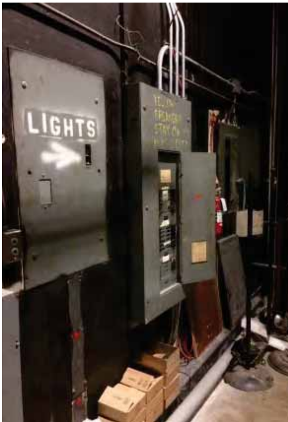
Existing unlabeled panel that should be replaced
