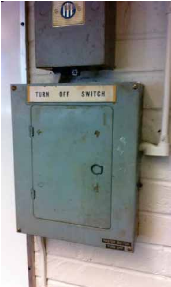
Existing panelboard, original to building
