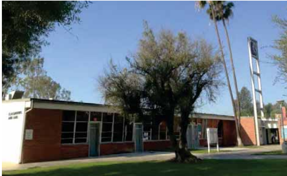
Figure 1C-6: North façade of Building 7 east wing with classroom door openings inserted into the angled glazed wall. The straight brick-clad shear wall is at the left and the clock tower at the right is attached to the brick-and-stucco restroom projection.
