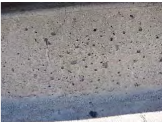
Figure 226: Concrete displaying a high level of air voids on the east bleachers and a vertical crack.
