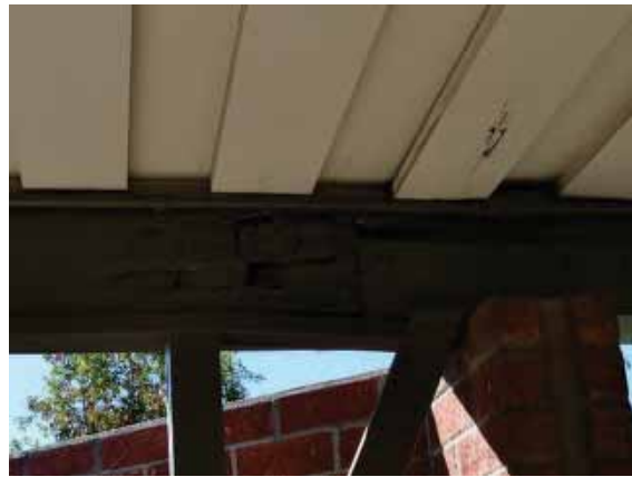
Figure 139: Rotten wood soffit and ceiling wood finish on the walkway canopy at Building 12.
