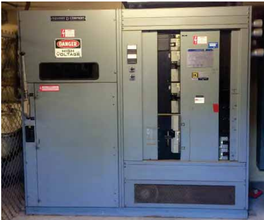
Existing unit substation
