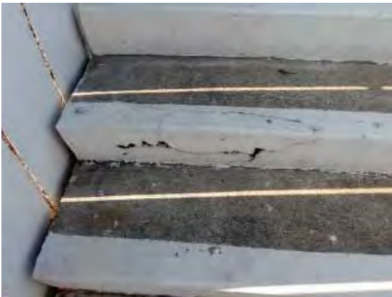
Figure 207: Insignificant spall on the left-hand steps.
