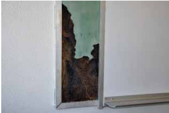
Figure 125: Damaged chalkboard behind modern white board in Room 111, Building 9.
