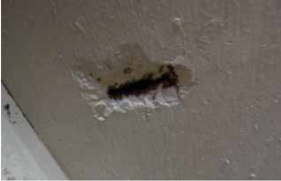
Figure 211: Spalled concrete related to oxide jacking of the rebar.
