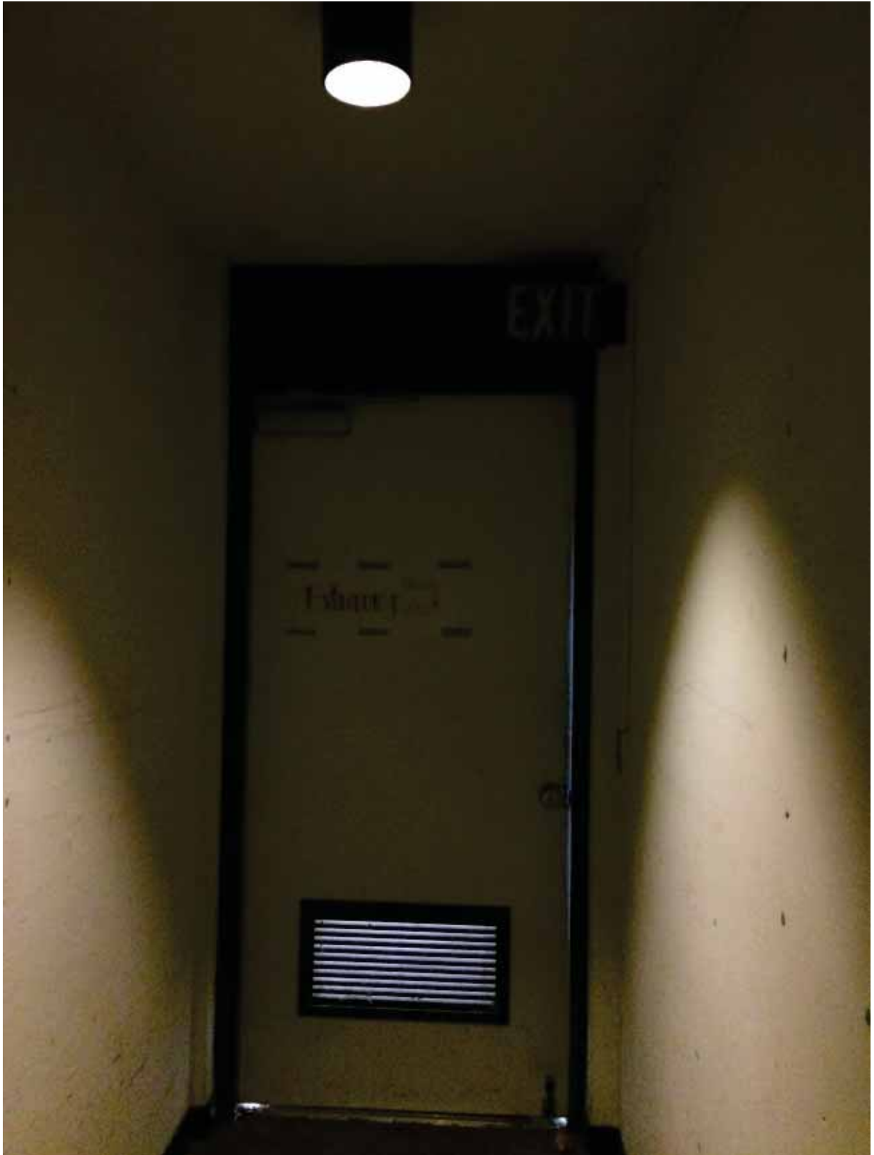
Existing aged self illuminated exit sign
