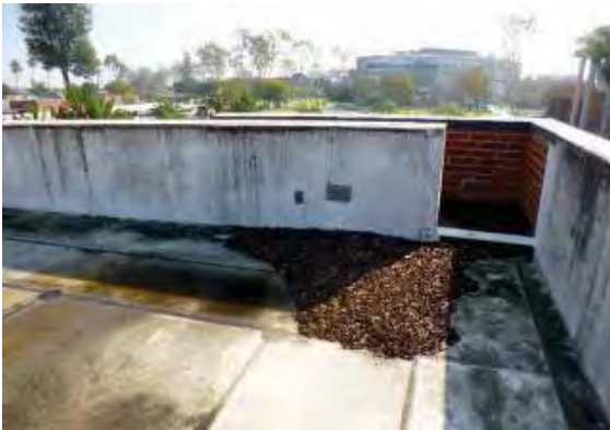
Figure 176: Soiling and heavy algal growth on the parapet walls of Building 37 plus accumulation of plant detritus.
