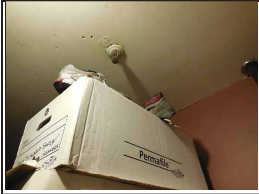
Photograph 1: Storage close to the sprinkler head in the fire sprinkler riser room in Building 2
