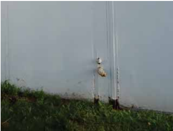
Figure 104: Corrosion at the base of the concrete channels between tilt-up concrete panels on the west façade of Building 7.
