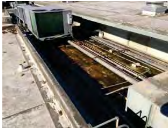
View of standing water next to HVAC unit
