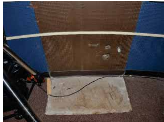
Figure 187: Removal of equipment has left areas of the flooring and pegboard wall finish lacking current paint finish and carpet.
