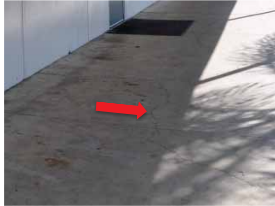
Figure 118: Cracks in the concrete slab neighboring Building 9.
