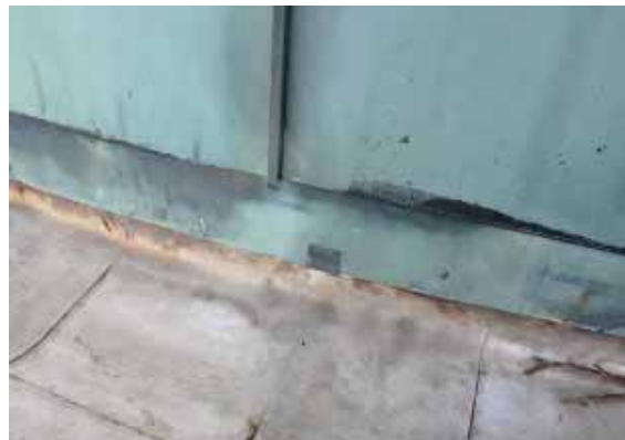
Figure 179: Corrosion visible below the copper flashing on the Planetarium (Bldg.39).
