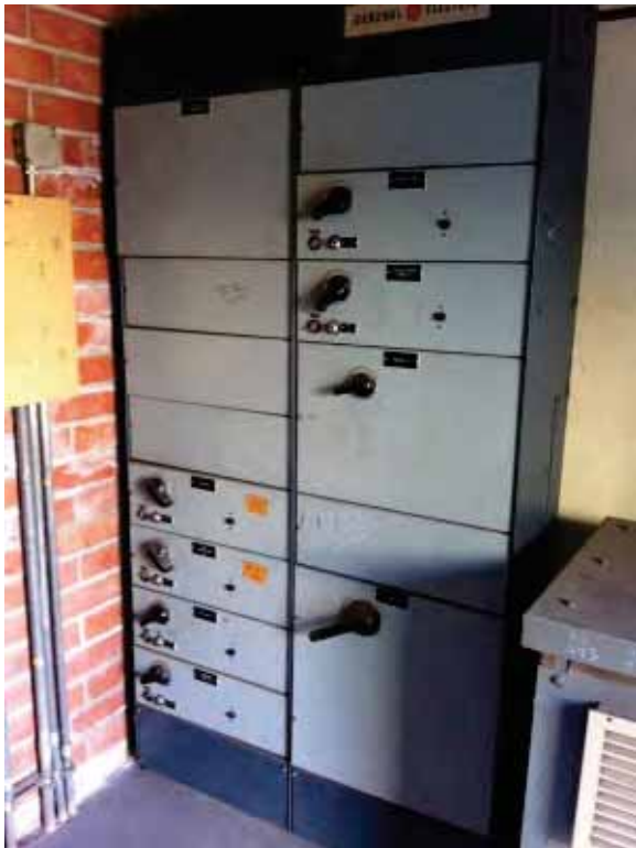
Existing Motor Control Center
