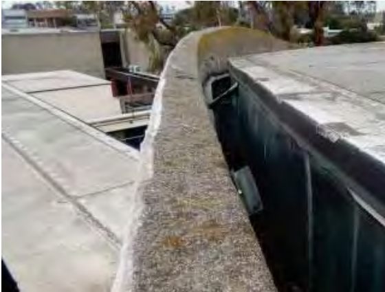
Figure 150: Widespread lichen growth (yellow) on the auditorium (Bldg. 2) parapet wall.
