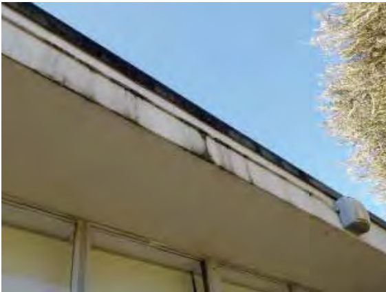
Figure 115: Soiling and algal growth on the north façade of Building 8.
