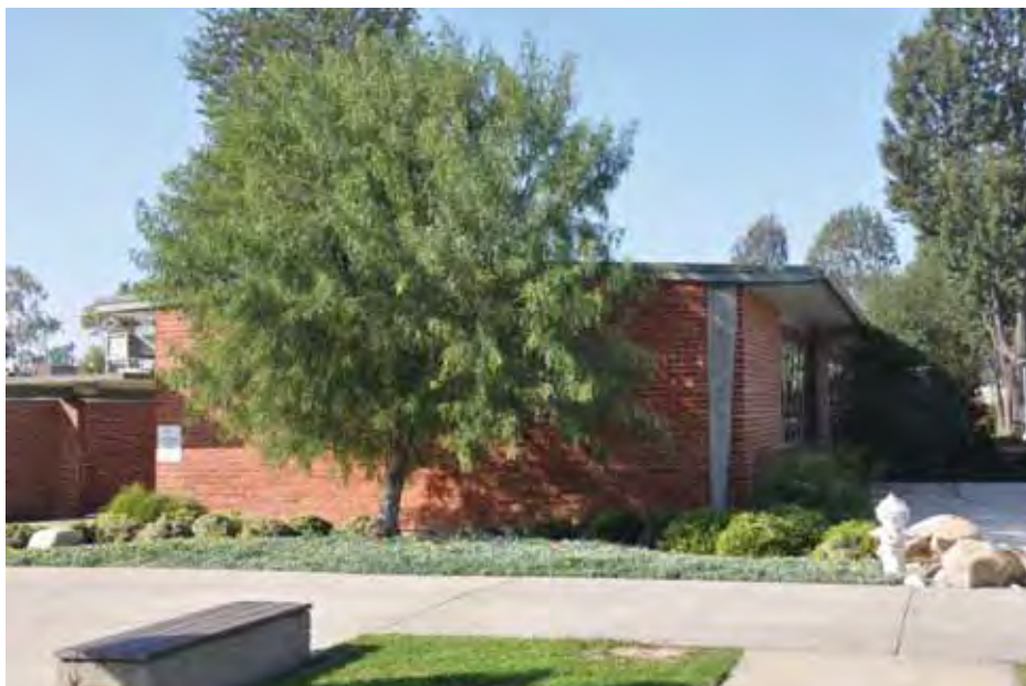
Figure 1C-35: East end of Building 12 with tapered aluminum section to transition from the north façade's angled wall. Brick-clad shear wall for seismic retrofitting seen here on the north façade.
