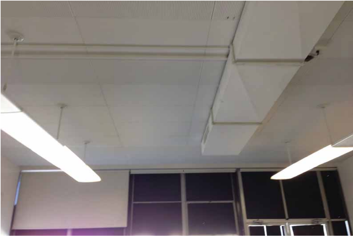
Photograph 5-General view of the suspect interior building materials, including ACM, LBP, light ballasts and mercury
