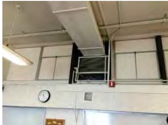
Ductwork within the classroom
