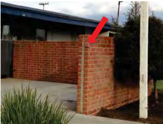
Figure 233: Brick wall at the south of the Field House with area of mortar missing visible.
