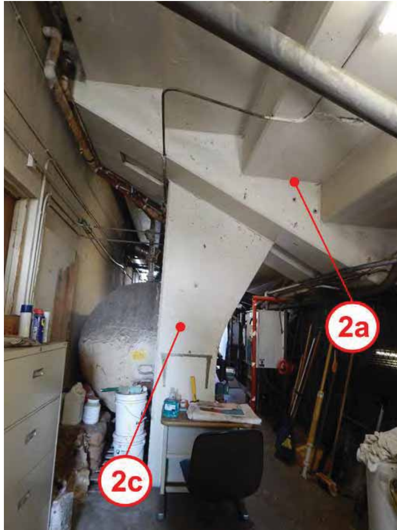
Figure 1D-32: Contemporary image below the Bleachers (Bldg. 93) with character defining features identified by red callouts.
