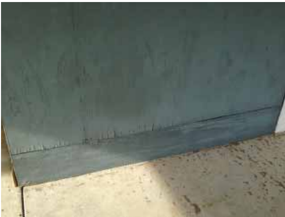
Figure 169: Water damage at base of plywood wall on east façade of Building 35.
