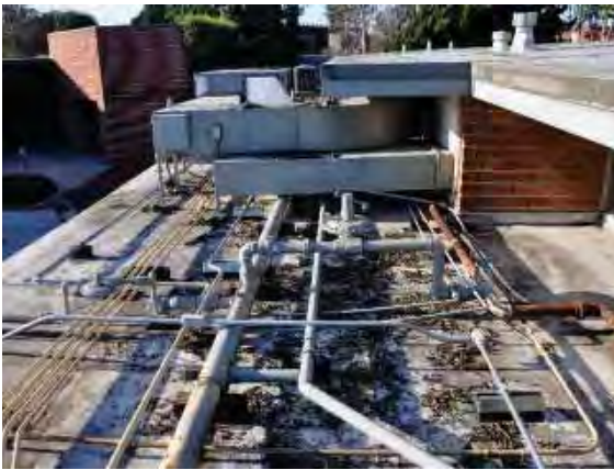
Figure 138: Network of pipes on the walkway canopy roof neighboring Building 12 with a build-up of plant detritus.
