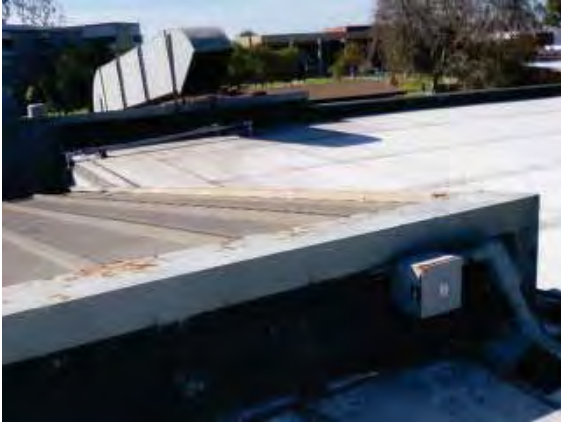
Figure 113: Plant detritus accumulation and paint peeling from the metal roof on Building 7.
