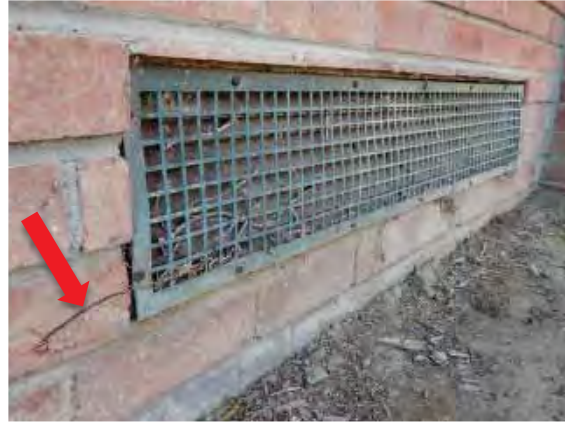
Figure 103: Integrated vent on the north façade of the east wing of Building 7 with fractured brickwork.
