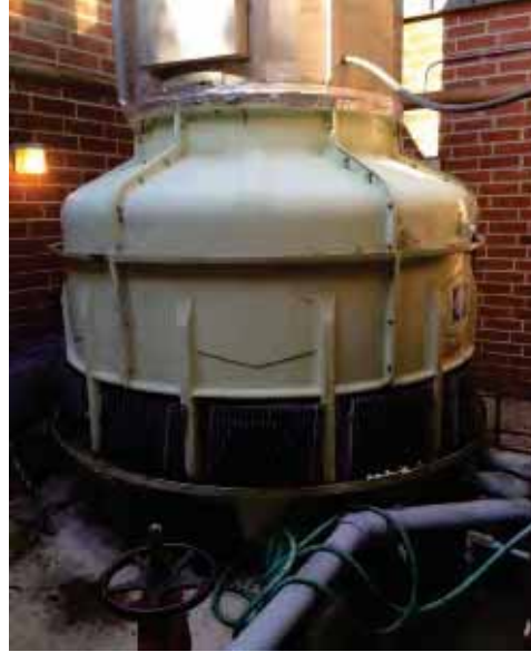
Fiberglass cooling tower
