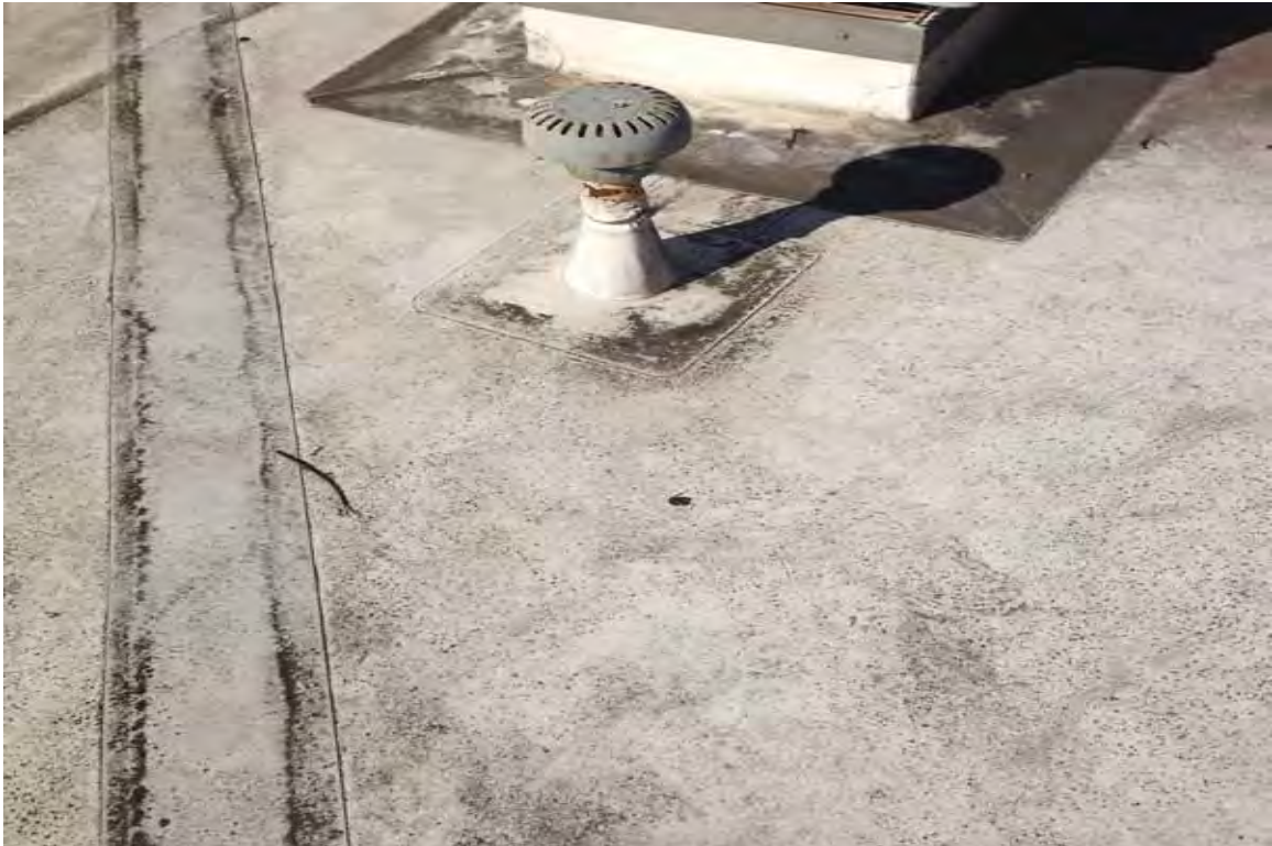
Photograph 14-View of the suspect roofing materials
