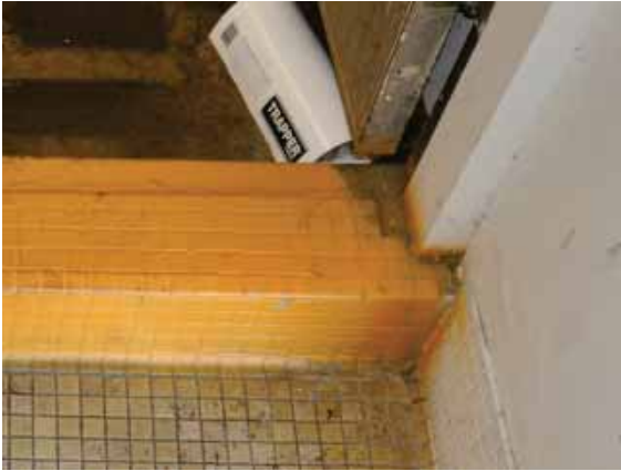
Figure 245: Rusting at the base of door, Field House, Building 110.
