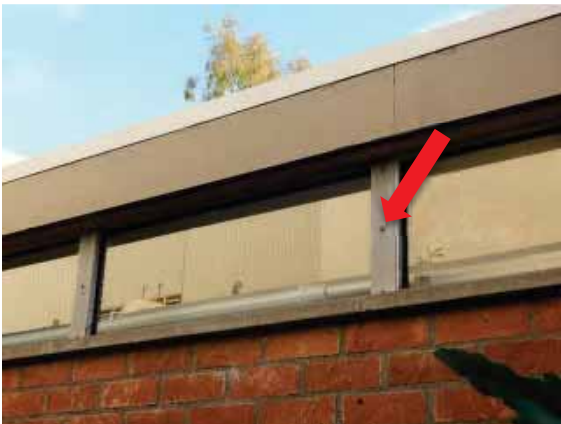
Figure 154: Clerestory windows on the west offshoot from Building 2 with corroded fasteners.
