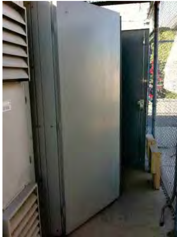
Existing 750kVA substation at exterior yard
