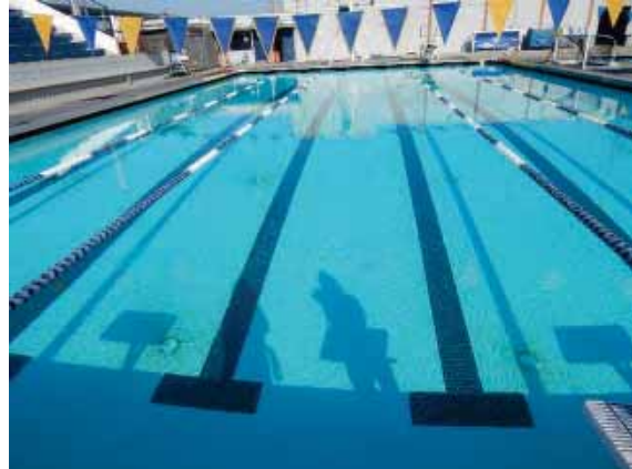
Figure 202: Staining around the edges of the filters in the base of the large pool.
