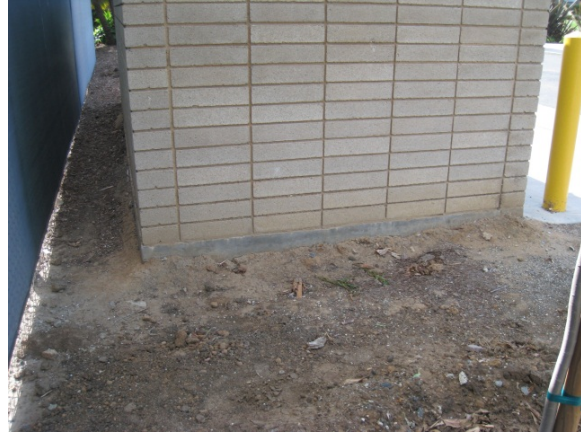
Figure 9. Same location as Figure 6. Close up of utility building with exposed ground surface at the base.
