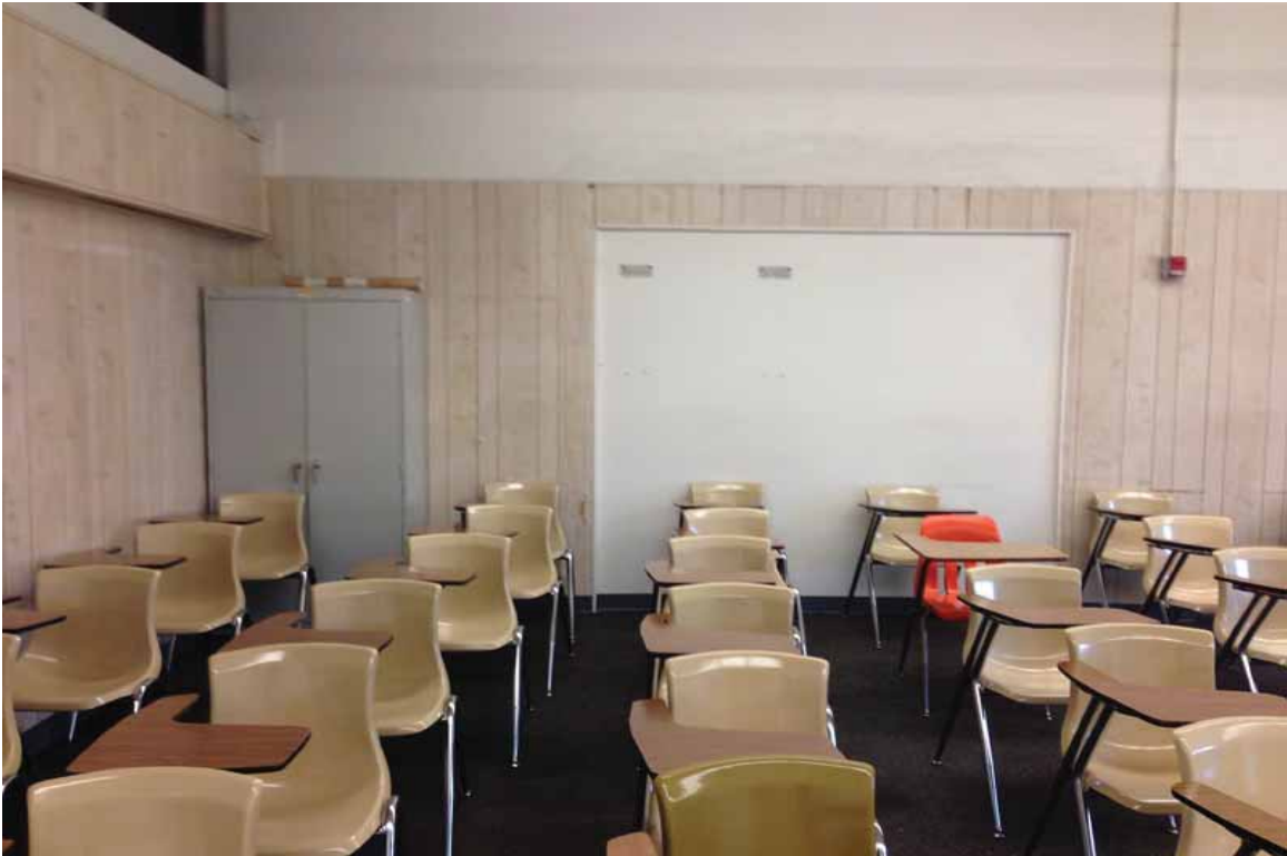
Photograph 3-General view of the suspect interior building materials
