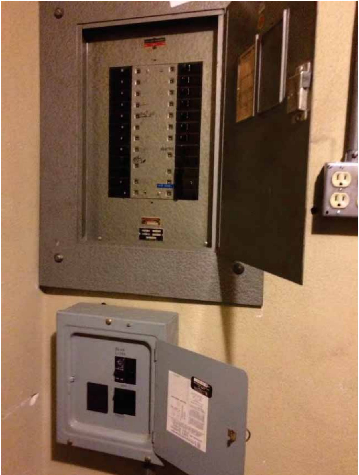
Existing panelboard original to building and load center mounted below
