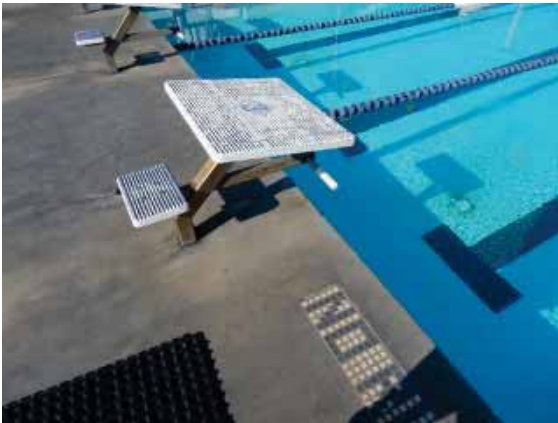
Figure 203: Corrosion on the starting platforms of the large pool.
