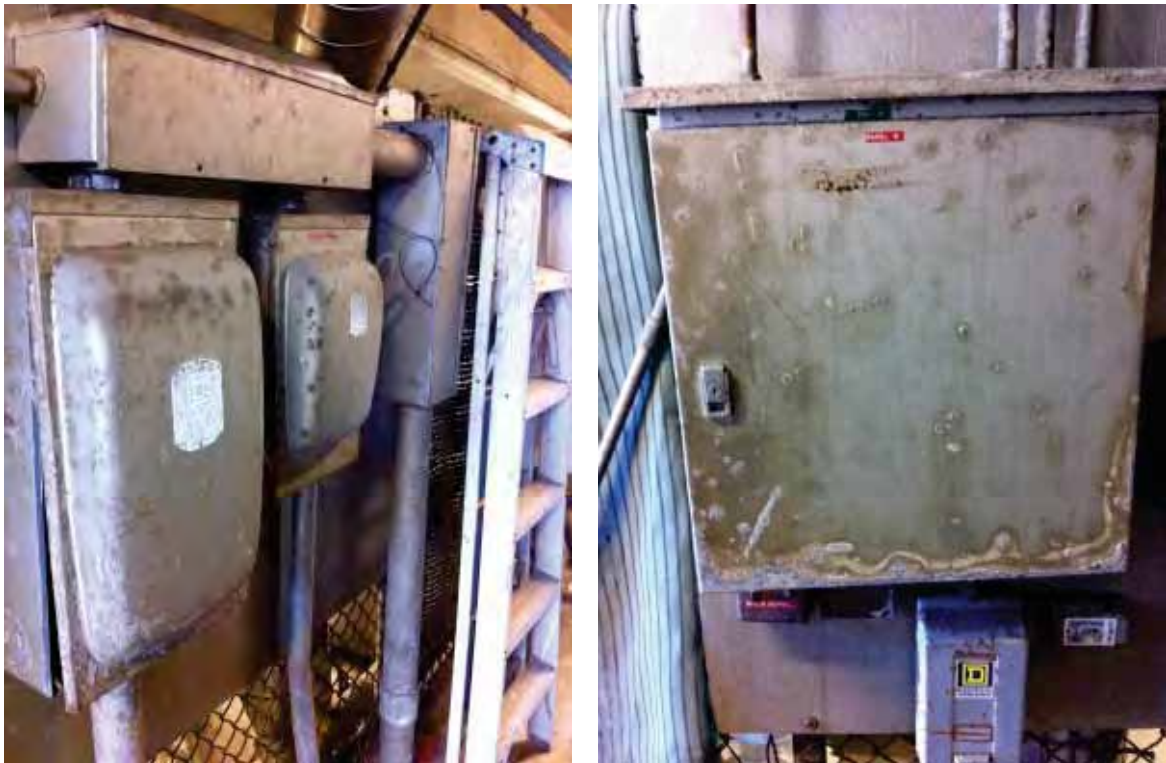
Existing electrical equipment and panelboard showing signs of corrosion
