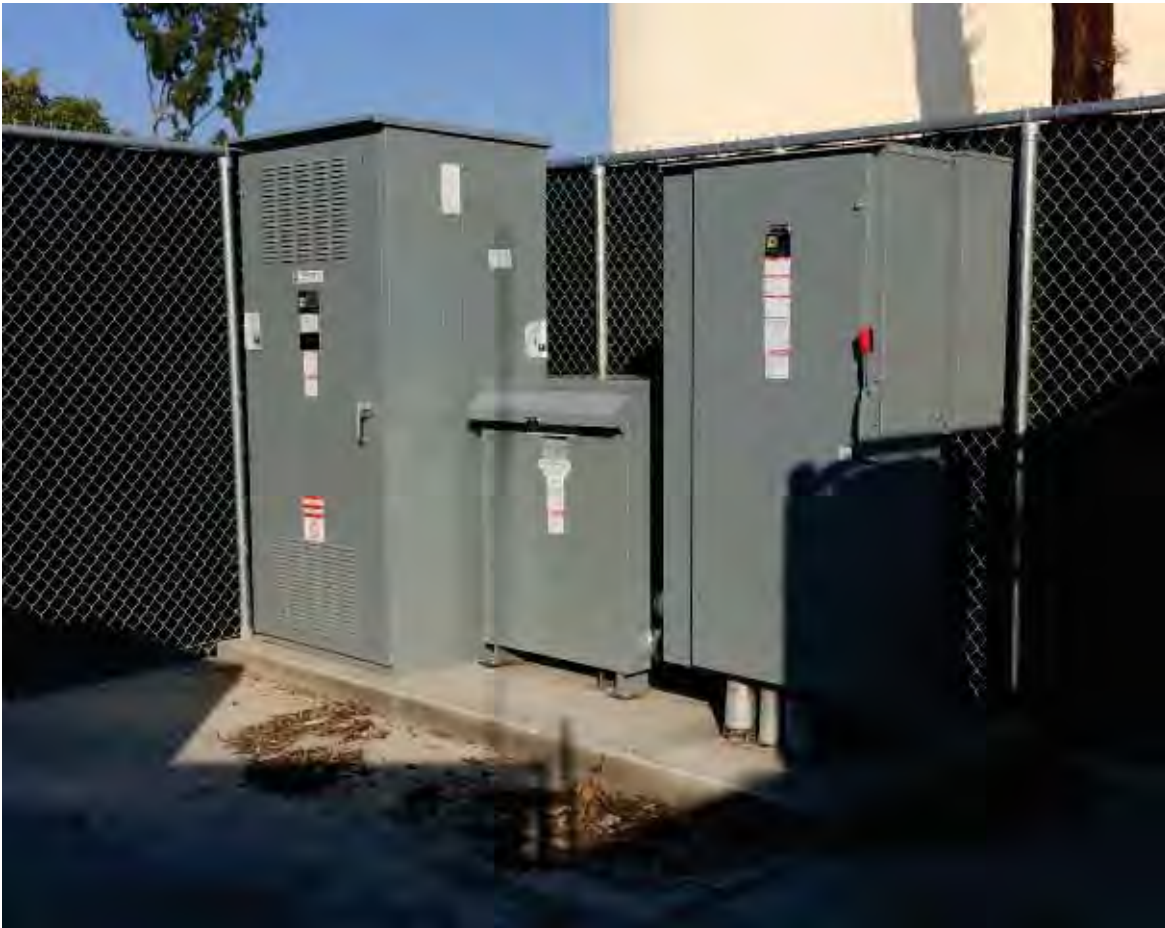
Exterior electrical yard between buildings 2 and 4 – 5kV switch, Transf. TVHM and Swbd STH
