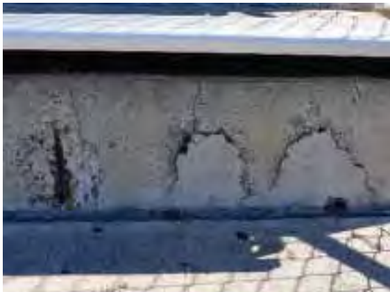
Figure 220: Corroded rebar causing oxide jacking and concrete spalling on the east bleachers.
