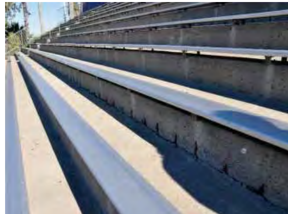
Figure 221: Vertical reinforcement visible and corroded along a whole level of the section north of center on the east bleachers.
