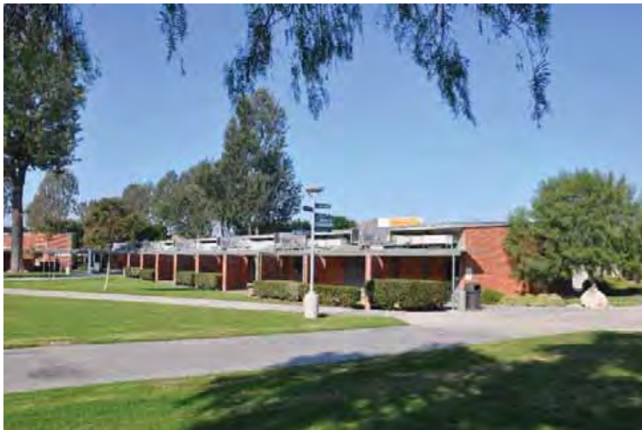
Figure 1C-39: Building 12's south façade with clerestory windows concealed behind HVAC equipment on the covered walkway, which is supported by angled brick wing walls at this side. The building's brick east façade is also visible.
