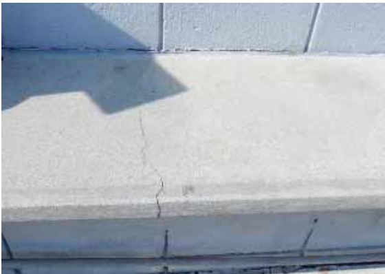
Figure 195: Hairline crack in the concrete bench on the east side of the pony wall.
