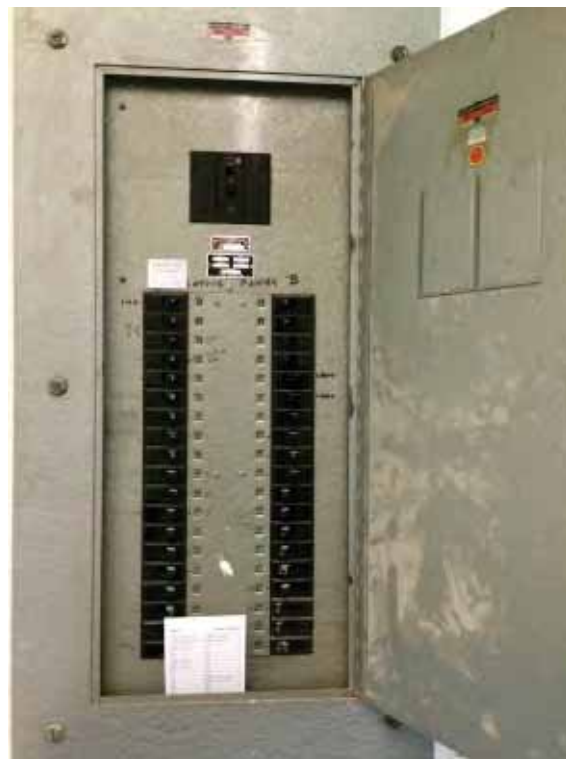
Existing panelboard original to building
