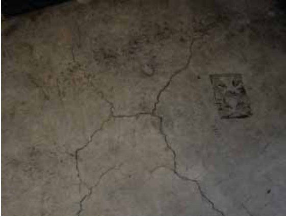
Figure 243: Cracking and crazing on concrete slab floors, Field House, Building 110.
