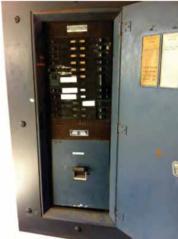
Existing panelboard at score booth
