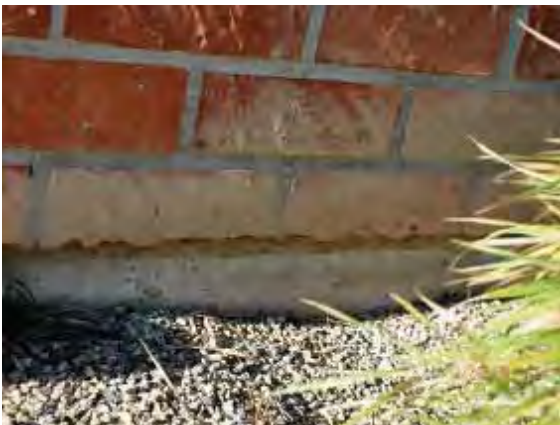
Figure 127: Chipped brick at the base of the east façade of Building 12.
