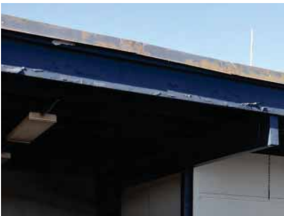
Figure 237: Paint peeling from the flashing and soffit at the east end of the Field House.
