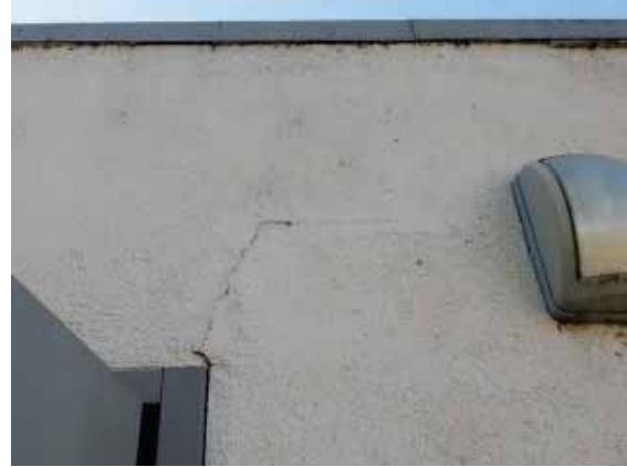
Figure 107: Crack at the top of the door frame on the north façade of the addition to Building 7.
