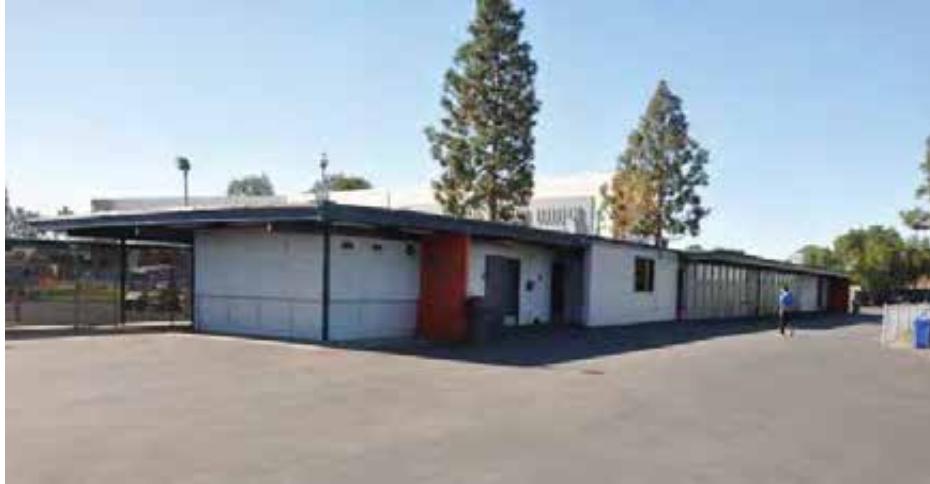
Figure 1C-108: North and east façade of Field House with deep roof overhang, looking southwest.
