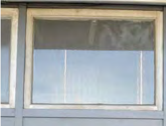
Figure 234: Dull patina on the aluminum window frames on north façade of Field House.
