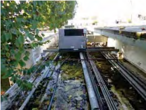
Figure 180: Accumulation of plant detritus and deep water pooling on the canopy roof of the walkway neighboring Building 36.
