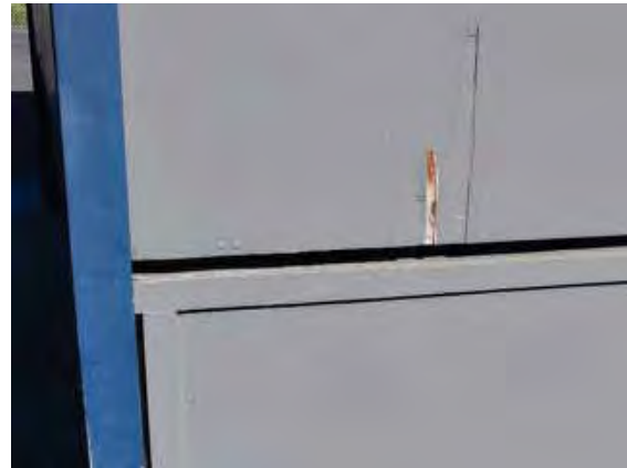
Figure 242: Small area of damage to plywood on west end of south façade.
