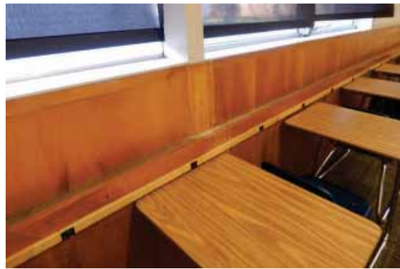
Figure 143: Plywood paneling with channel below the windows on the north wall in Room 101, Bldg.12.
