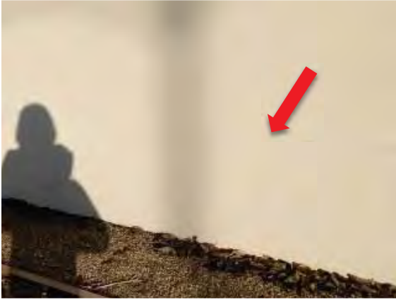
Figure 152: Horizontal crack on the west façade of the original (north) portion of the Music Building (Bldg. 2).
