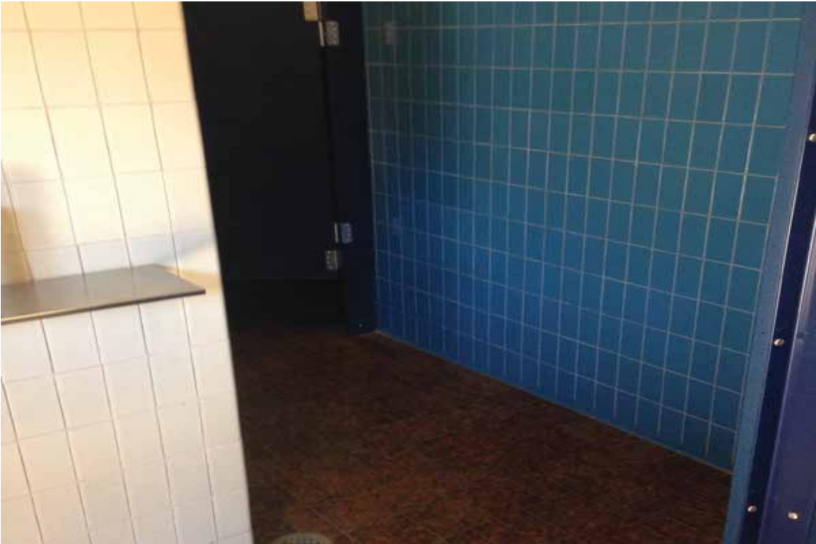
Photograph 6- View of the suspect lead ceramic tiles in the restrooms
