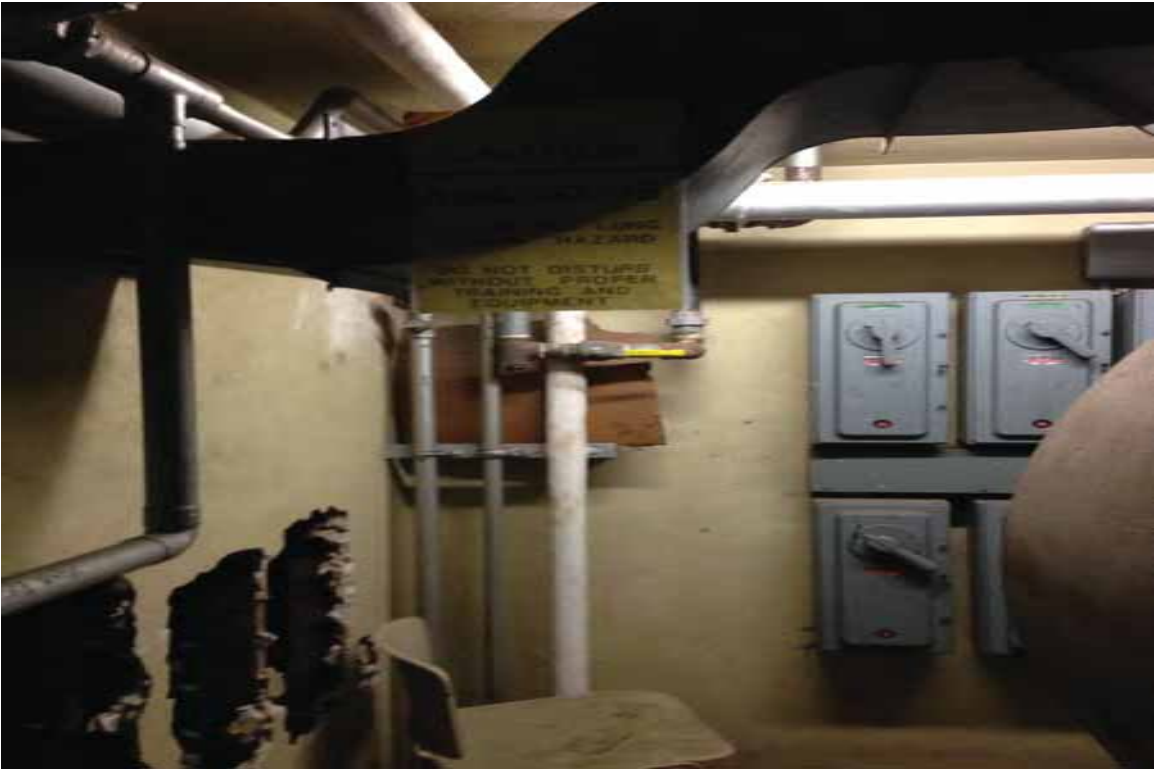
Photograph 7-View of pipe insulation inside the mechanical room
