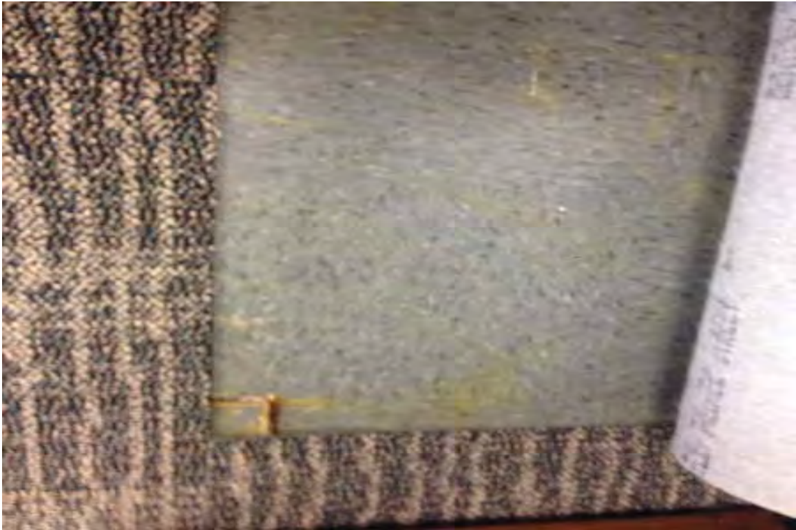
Photograph 8-View of suspect floor tile & mastic under carpet
