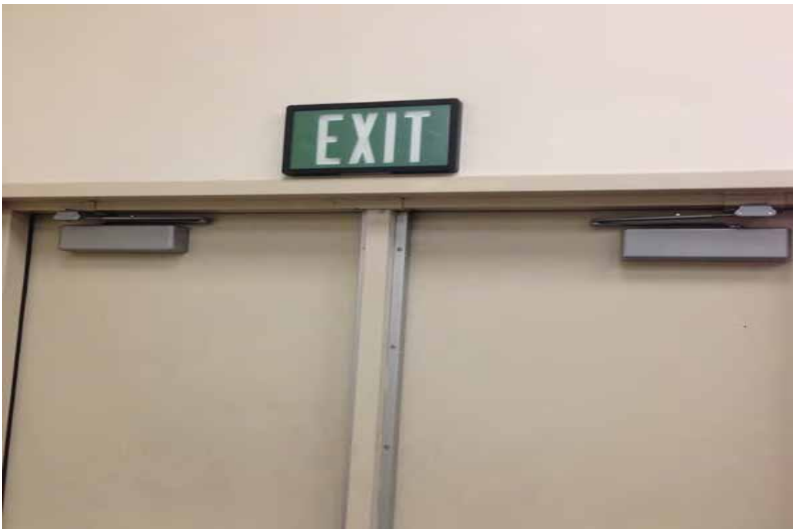
Photograph 14-View of the exit sign with suspect tritium gas
