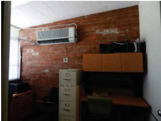
Figure 121: Efflorescence on exposed brickwork inside Office C, Building 8.
