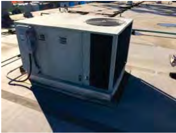
DX Heat Pump Unit
