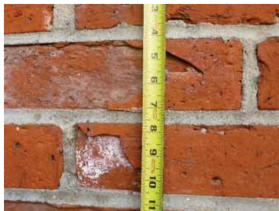
Figure 164: Spalling brickwork and efflorescence on east façade of Building 37.
