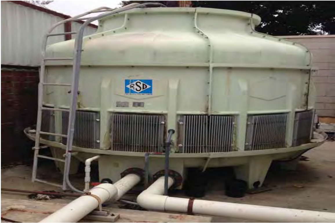
Photograph 15-View of the cooling tower with suspect insulation
