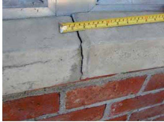
Figure 109: Cracked window sill on the north façade of Building 8.
