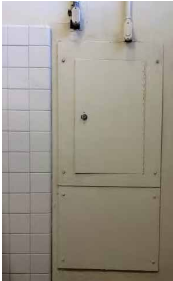
Existing panelboard, located in restroom
