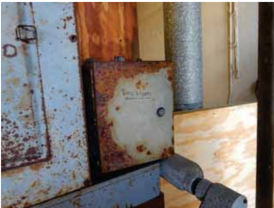
Figure 218: Corroded casing to pool lights controls.
