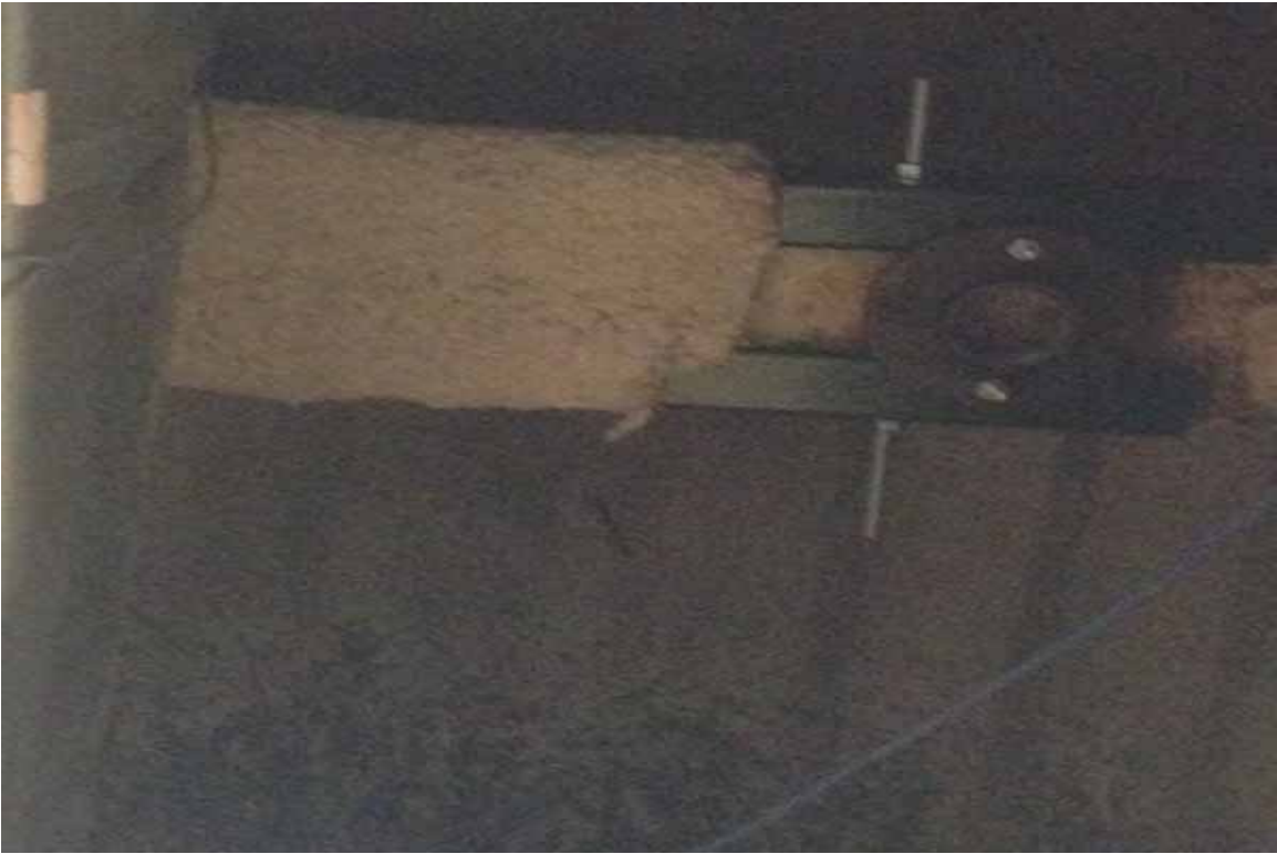
Photograph 10-View of the suspect fireproofing and overspray on beams
