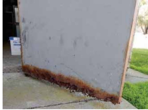
Figure 112: Heavy corrosion at the base of the door on the north façade of the addition on the west end of Building 7.
