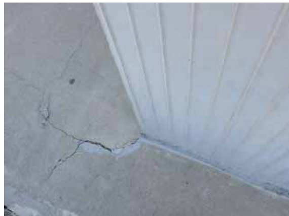
Figure 225: Localized area of cracking of the concrete slab at the top of the east bleachers.
