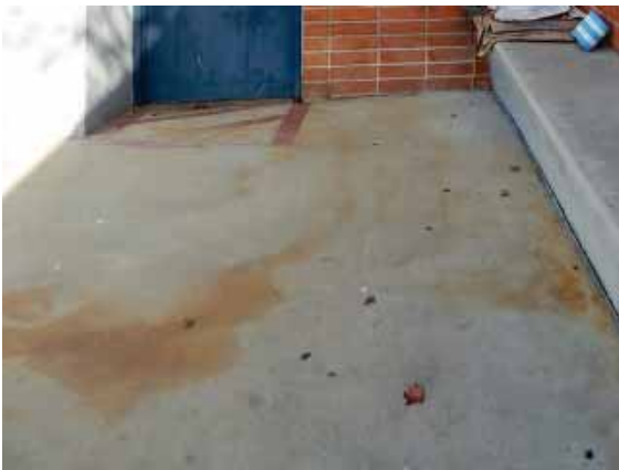
Figure 199: Oxide staining on the concrete slab paving at the north east corner of the complex.
