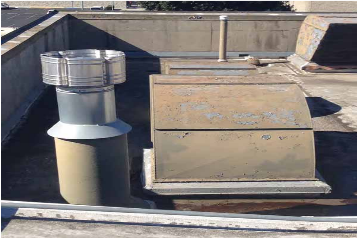
Photograph 10-View of the suspect transite pipe, roofing and lead paint materials
