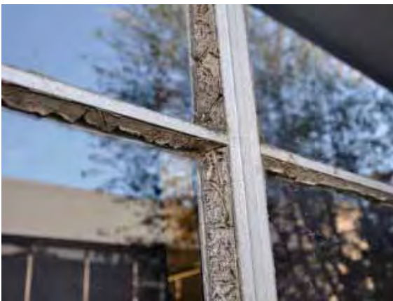
Figure 134: Deteriorated glazing putty as seen on the north façade of Building 12.
