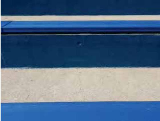
Figure 205: Cracking in the bleacher treads.
