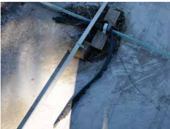
Figure 239: Remaining detached sheathing on the roof of the Field House.
