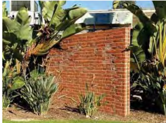
Figure 166: Spalling brickwork on a wing wall at Building 35.
