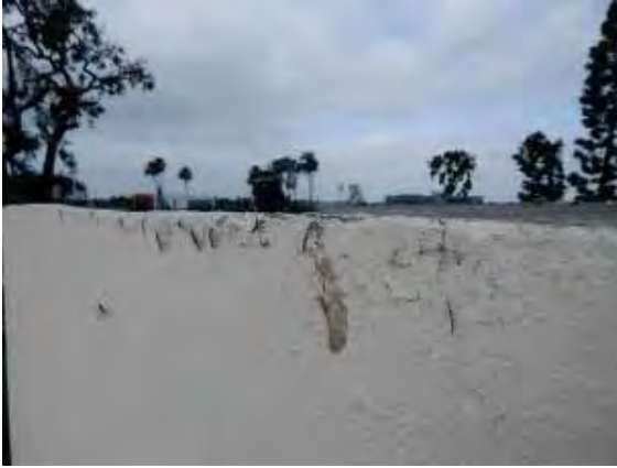
Figure 148: Crack on the west façade of Building 2 with textured finish and paint loss.
