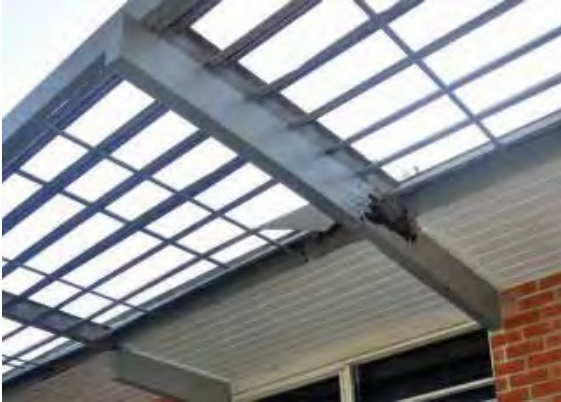
Figure 141: Rotten beam and damaged slat at the roof edge, plus stunted wooden beam in the background.
