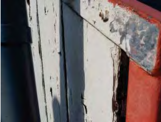
Figure 217: Outside of the railings and fence at the south side of the bleachers showing a loss of paint on the railings, peeling paint on the wood fence, and corrosion of ferrous fasteners.
