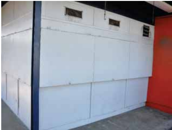
Figure 241: Soiling below the grills at the east end of the Field House.
