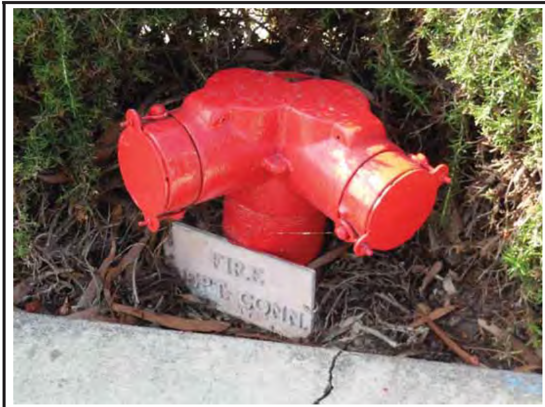
Photograph 4: FDC not identifying what buildings it serves. The picture also shows an improper cap on the FDC.
