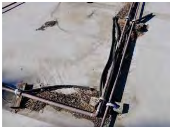
Figure 240: Accumulation of plant detritus around the conduits on the roof of the Field House.
