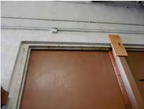
Figure 216: Corroded door frame on the east side of the west wall.
