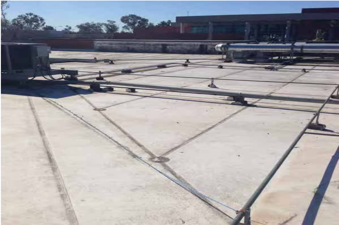
Photograph 13-General view of the suspect roofing materials
