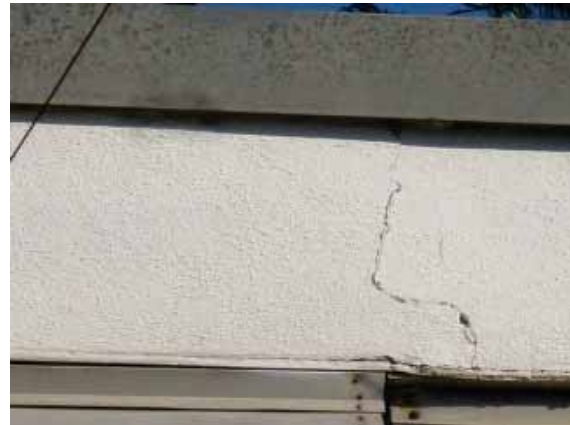
Figure 116: Crack running through the face of the soffit on the south façade of Building 8 at the line of the building addition.
