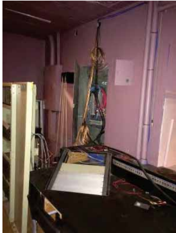
Existing unlabeled panel and unsupported cabling
