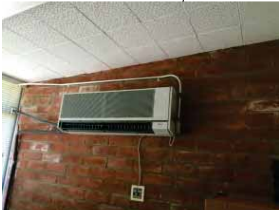
Ductless wall mounted Fan Coil
