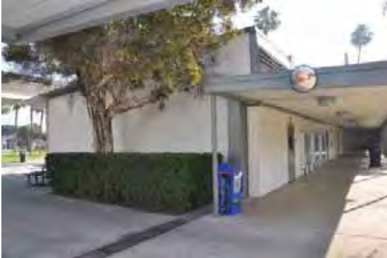
Figure 1C-24: Covered walkway and Building 8's west end at the patio, looking east.
