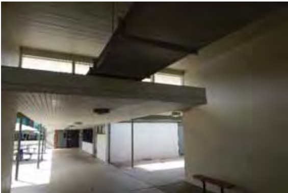
Figure 1C-91: Intersecting covered walkway in breezeway. Note the different ceiling treatments and the clerestory windows.
