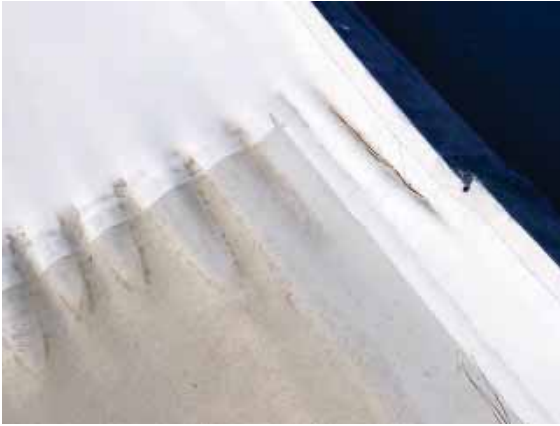
Figure 235: Buckling patch on roof and small hole in membrane at edge of roof at the center of the north side.
