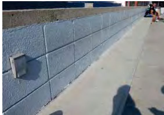
Figure 196: The joint between the pony wall and the top of the concrete bench is cracked along most of its length.
