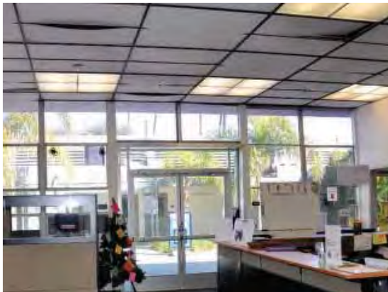
Figure 123: ceiling tile sagging and coming out of its framing in Room 103B, Building 7.
