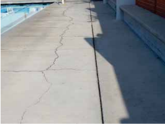
Figure 197: Cracking at the east side of the small pool.
