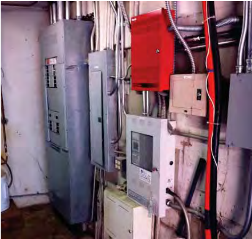
Building 7 Electrical Room – Water heater to left in front of Swbd
