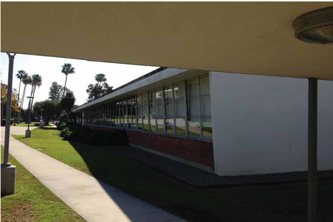
Photograph 2-General view of the suspect exterior building materials, including window putty and lead paint
