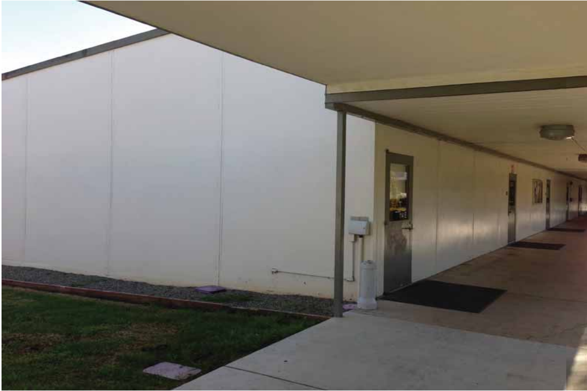
Photograph 1-General view of the suspect exterior building materials
