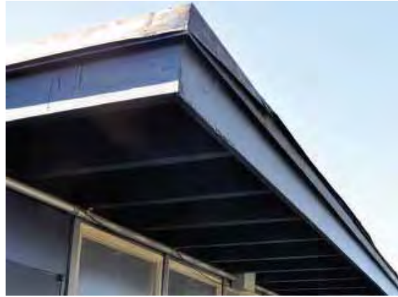
Figure 236: Displaced flashing on the north side of the building.
