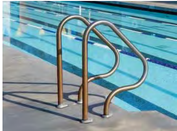
Figure 204: Tarnishing or corrosion on the entry handrail.
