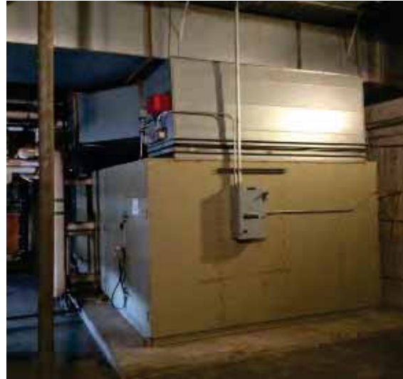
Custom Air Handler within Mezzaine
