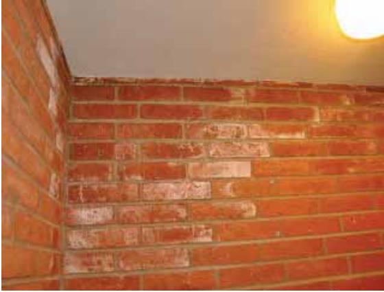
Figure 188: Efflorescence on internal unpainted brickwork in plan north hallway at Building 39.
