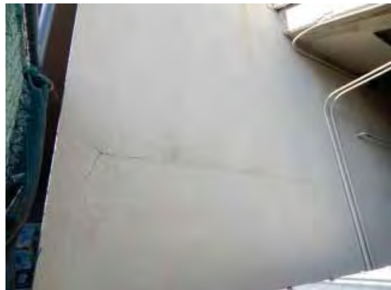
Figure 214: Crack on the south end of the east side of the wall.
