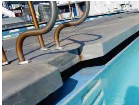
Figure 200: Concentrated oxide staining on the side of the slab by the entry hand rails at the south of the small pool.
