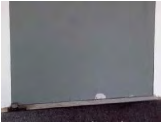
Figure 110: Door at the west end of the south façade of Building 9 with water damage to the base causing splitting and peeling paint.
