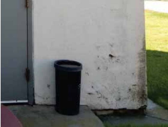
Figure 106: Blistered paint, soling and missing stucco on the north façade of the addition to Building 7.
