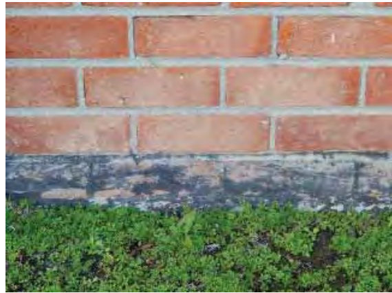
Figure 101: Deteriorating black painted damp proof course on the east façade of Building 7.
