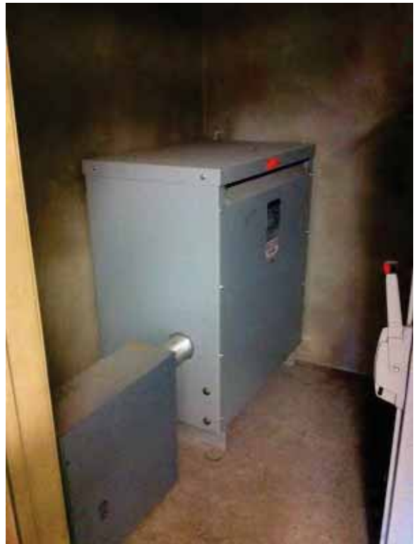
Existing transformer room without ventilation
