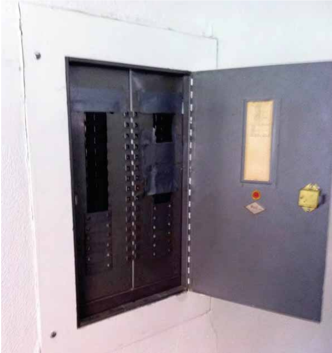
Existing Zinsco Panelboard Original to Building
