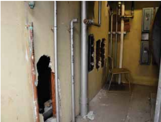
Figure 186: Large holes broken into the south wall of the mechanical room at Building 37.
