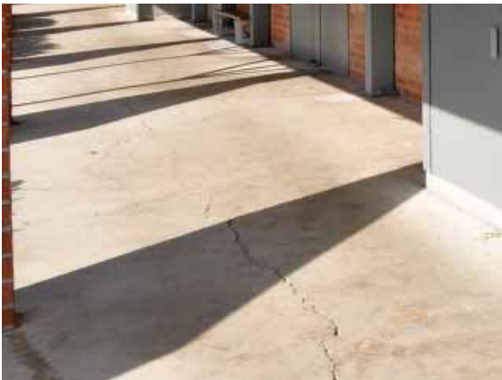
Figure 140: Crack in the concrete paving slab below the covered walkway at Building 12.
