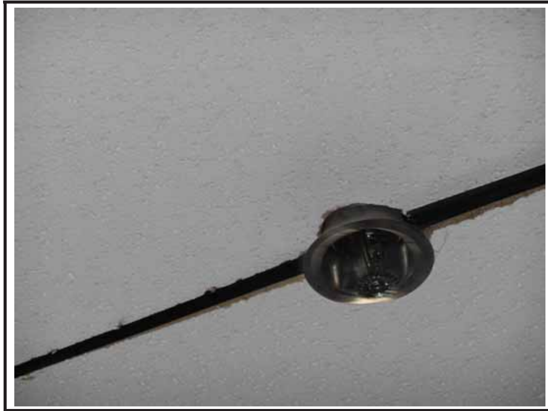
Photograph 7: Building 7 ceiling tiles warped so the fire sprinkler escutcheon won't go flush against the ceiling.
