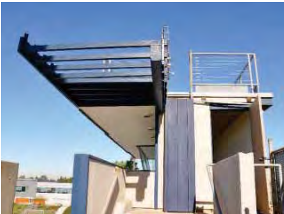
Figure 230: Gap in the railings at the south end of the east press box roof posing fall hazard.
