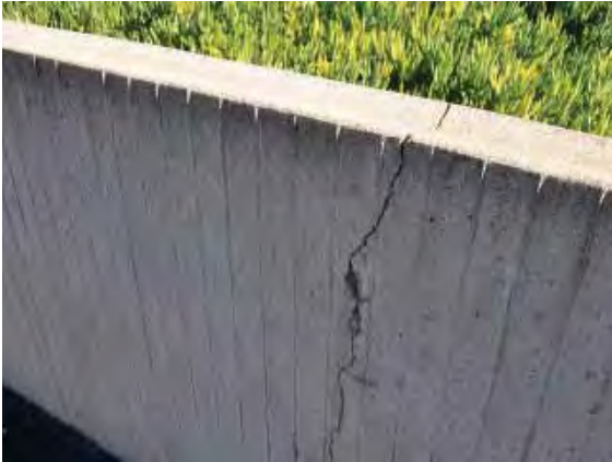
Figure 231: Crack running through a low wall on the east side of the stadium south of the bleachers.
