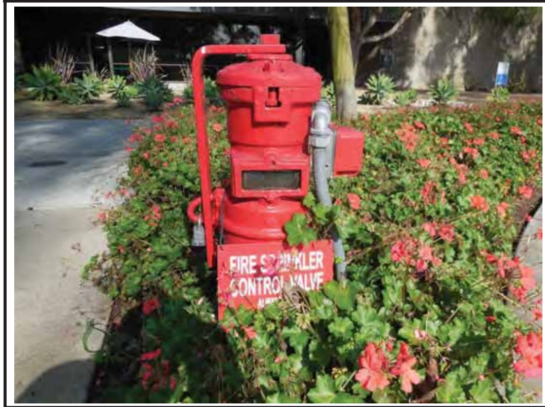
Photograph 5: Unable to read PIV to determine if the valve is open or closed.
