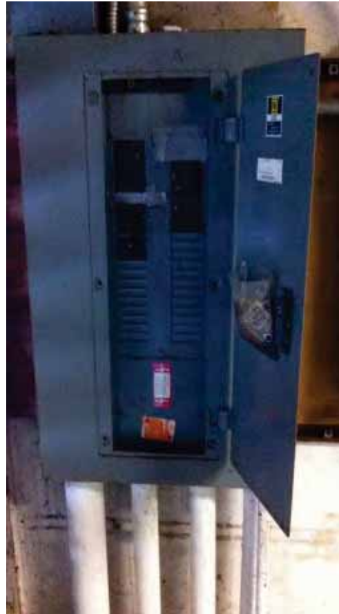
Existing panelboard, original to building
