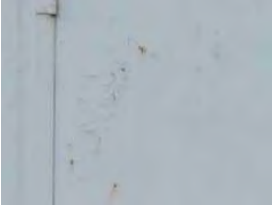
Figure 111: Corrosion showing through the paintwork on the steel door on the east façade of Building 7.
