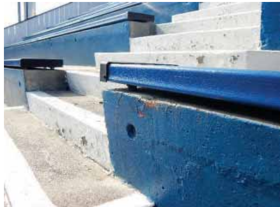
Figure 208: Crack at the corner of a seat possibly related to the fixture above.
