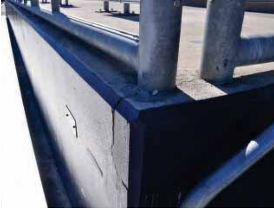
Figure 222: Cracking at a corner of the west bleachers associated with the railings fixtures.
