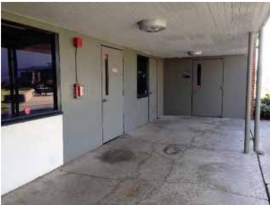
Figure 182: Cracking and oxide staining on the concrete paving slabs on the west side of Building 37.
