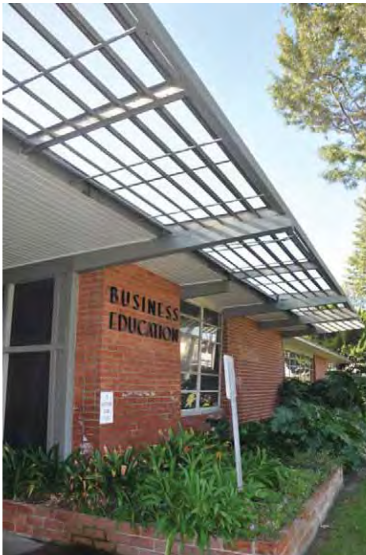
Figure 1C-32: The metal trellis on the north side of Building 13 at the breezeway.
