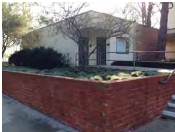
Figure 1C-56: North (left) and west (right) façade of Building 2B. Note the north half of the building is an addition with stucco cladding. The brick planter is part of the complex's landscaping.
