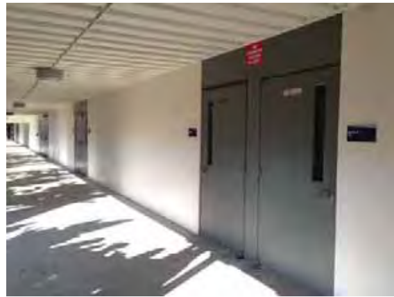
Figure 1C-73: Typical plywood surrounds around some doorways in Building 35 and 36. Note the wide board and batten ceiling of the covered walkway.
