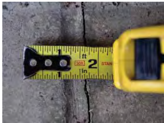
Figure 135: Crack at join between window sill units.
