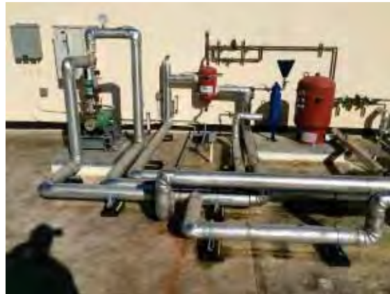
Boiler piping and equipment
