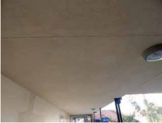
Figure 158: Cracking in the ceiling of the north-south walkway neighboring Building 4.
