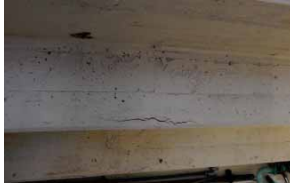
Figure 212: Cracked area with the potential for material loss.
