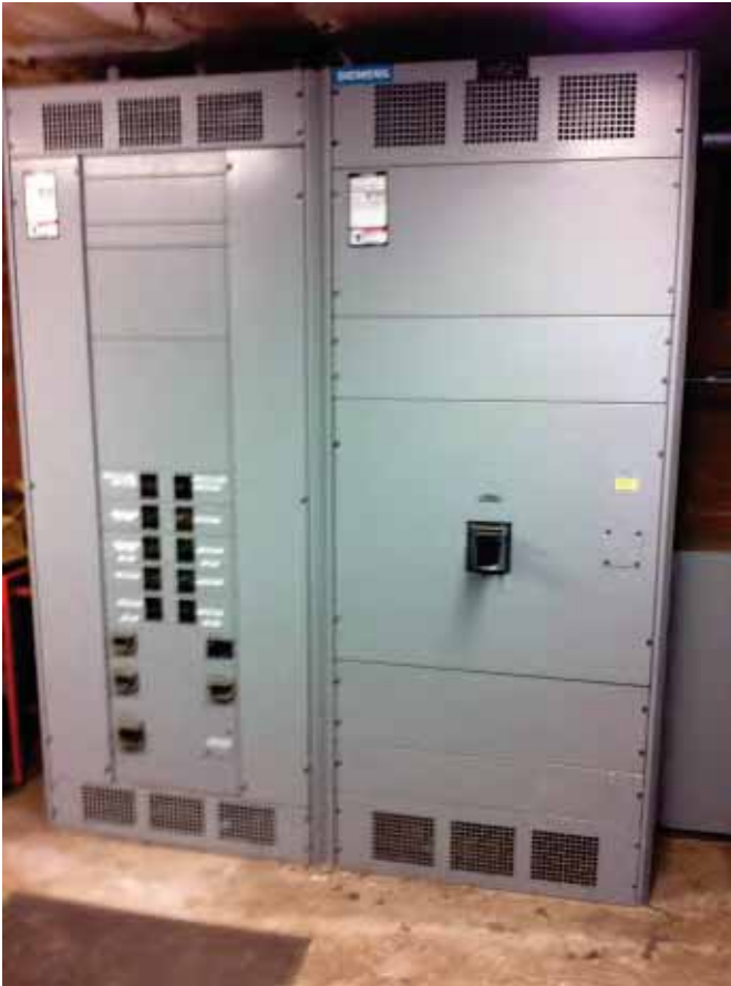
Existing Distribution Board DPS
