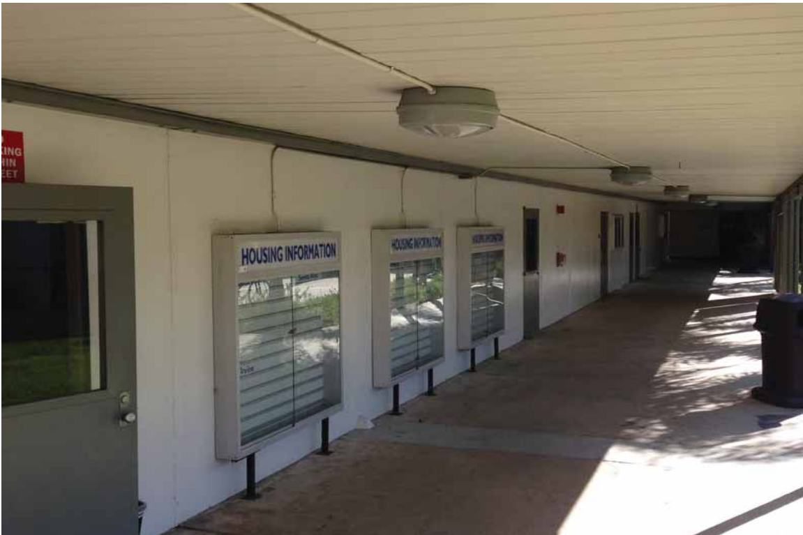
Photograph 2-General view of the suspect exterior asbestos and lead containing materials
