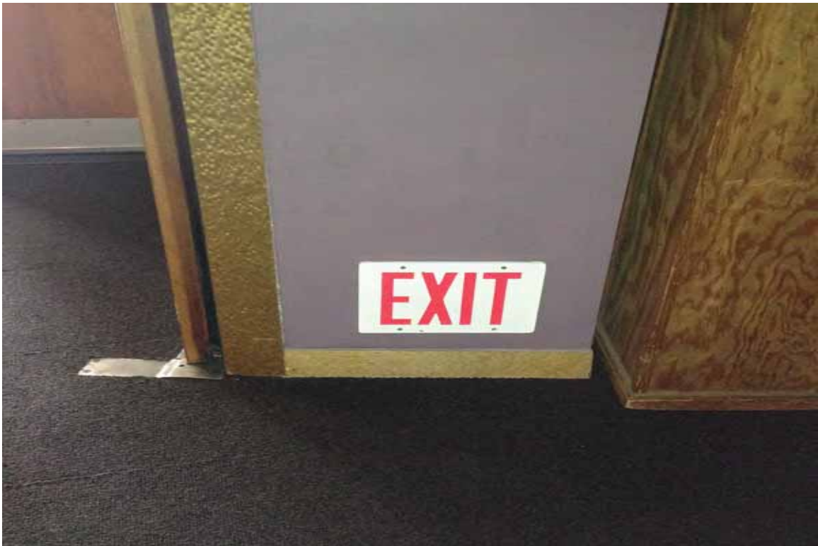
Photograph 6-View of the exit sign with suspect tritium gas
