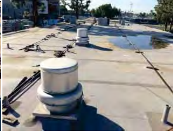
Exhaust Fans from Restrooms
