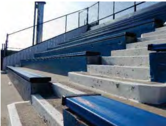
Figure 209: Peeling paint on the risers of the steps.
