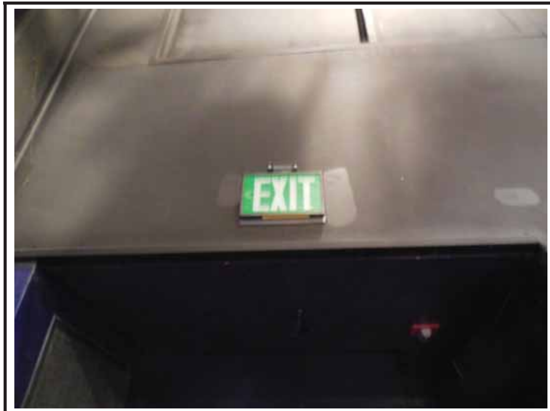
Photograph 6: Exit sign in the Drama Rooms not lit up.
