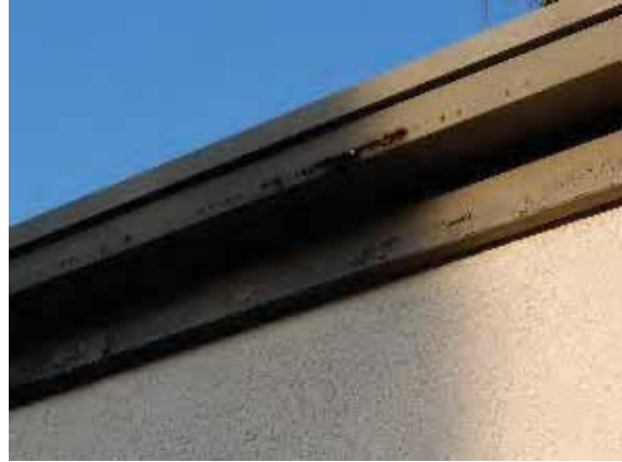
Figure 114: Heavily corroded gutter on south façade of east wing of Building 7.
