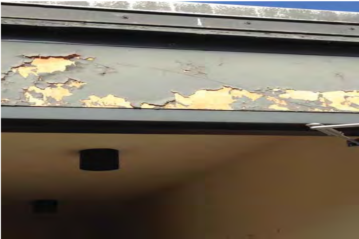
Photograph 13-View of exterior peeling paint
