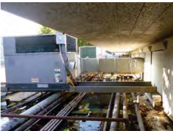
Figure 172: Mechanical equipment on the walkway canopy roof connected to the interior through modified clerestory windows on Building 36.
