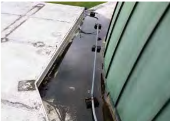
Figure 178: Water accumulation on the east side of the Planetarium (Bldg. 39) flat roof surrounding the copper dome.
