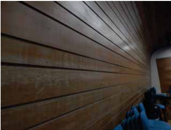
Figure 160: Original wood-paneled back wall and ceiling showing signs of wear in Room 101, Music Building (Bldg. 4).
