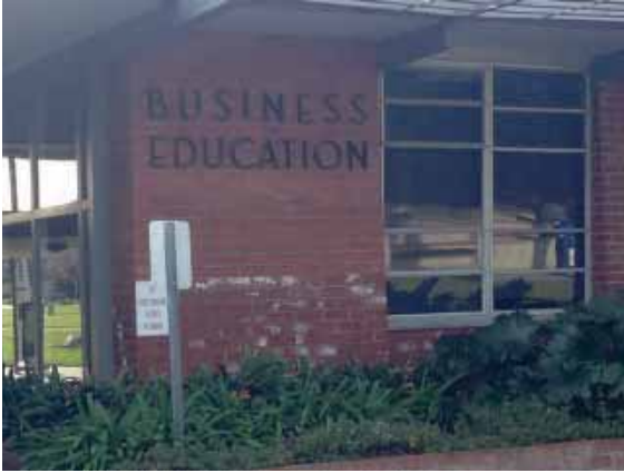
Figure 129: Heavy efflorescence on the north façade of Building 13.
