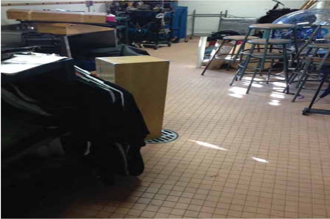
Photograph 14-View of suspect lead containing ceramic tiles & drain
