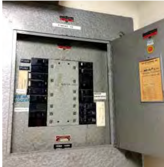
Existing panelboard original to building
