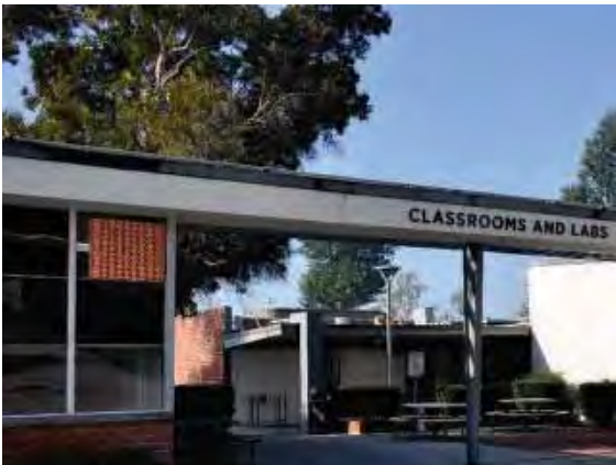
Figure 119: Algal growth and light soiling on the flashing and stucco sides of the trellis and boxed eaves between Buildings 8 and 9.
