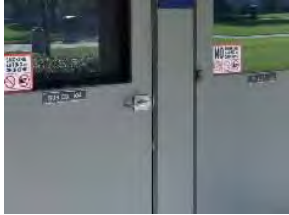
Figure 133: Chipped paint at the edges of the plywood side panel.
