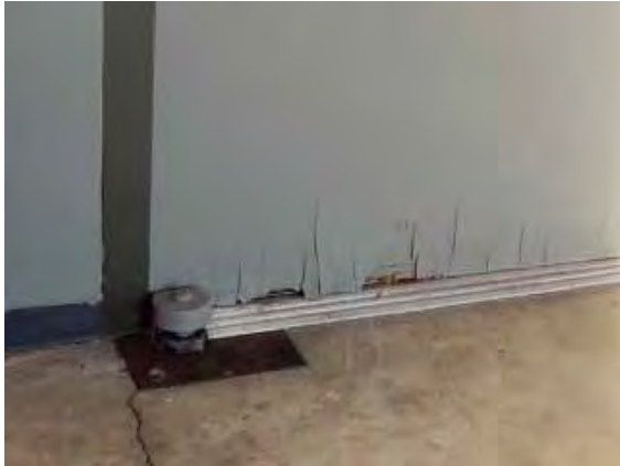
Figure 136: Water damage at the base of a wood door on Building 12.
