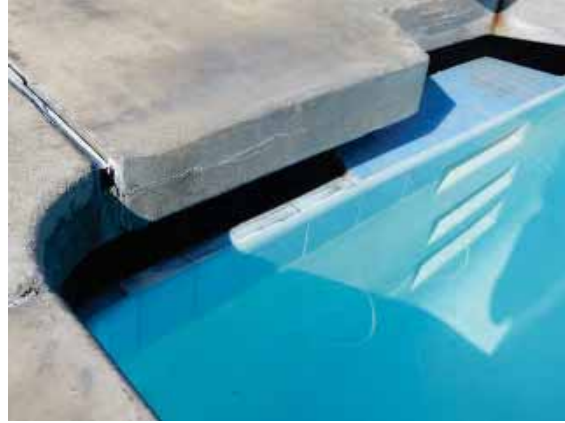
Figure 198: Crack on the side of the slab overhanging the integrated gutter at the southwest corner of the small pool.
