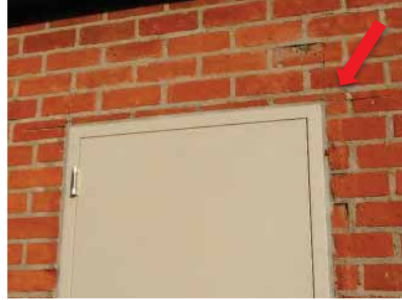
Figure 147: Cutting lines through the brickwork at the location of a new door insertion on the west façade of the Music Building (Bldg. 4).
