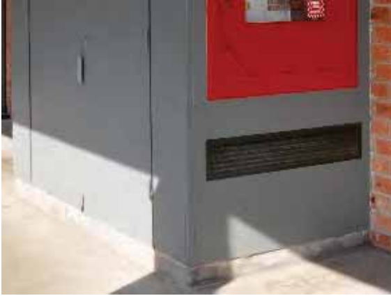
Figure 132: Water damage at the base of the plywood external storage units on Building 12.
