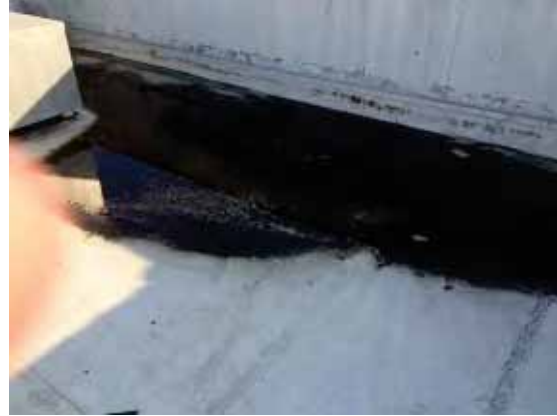
Standing water next to Multizone Unit
