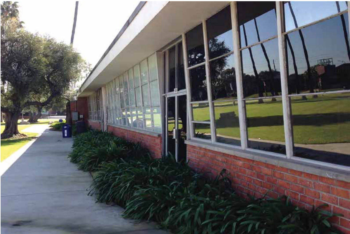
Photograph 3-General view of the suspect exterior building materials
