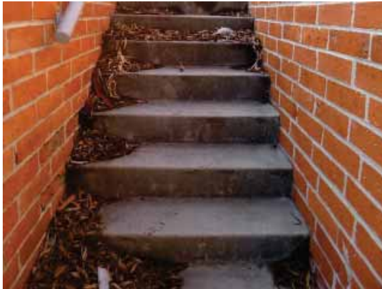
Figure 183: Plant detritus on the external stairs of Building 37 above the gate.
