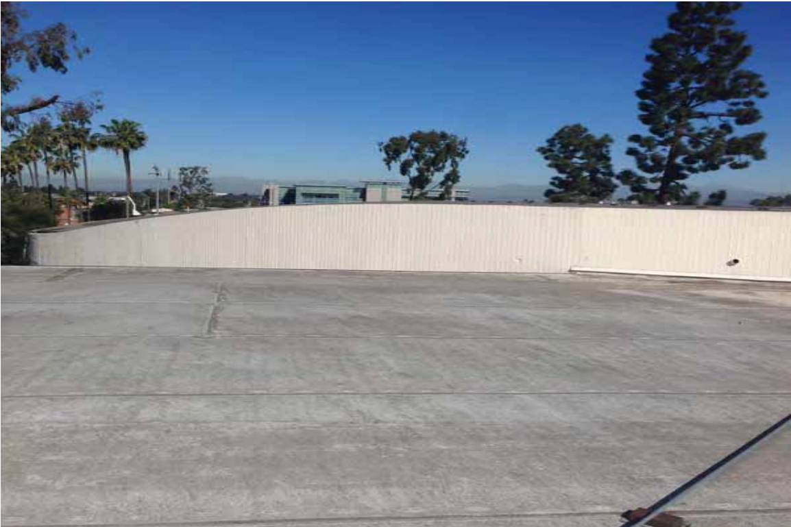
Photograph 8-General view of the suspect roofing materials
