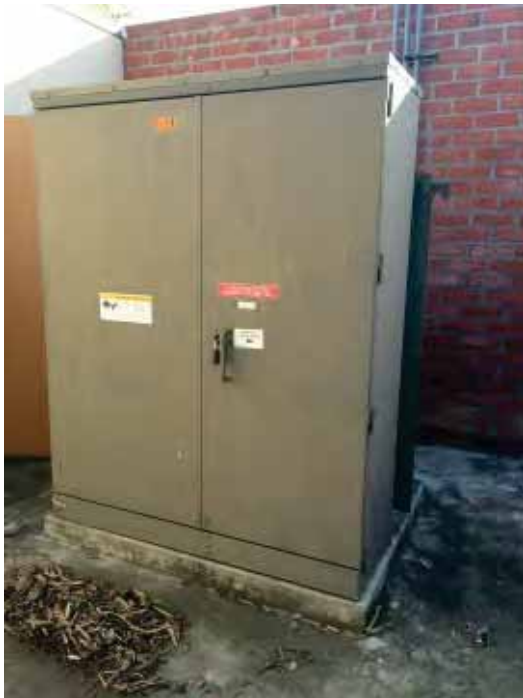
4160V Transformer T-24
