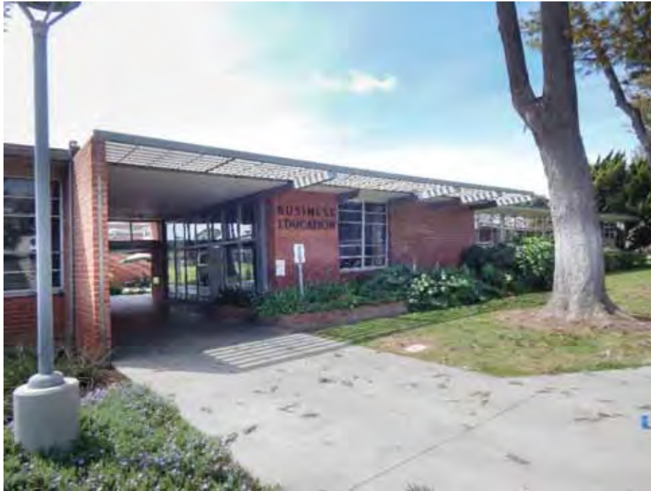
Figure 1B-24: Breezeway between Buildings 12 (left) and 13 (right) with shear walls added on north façade.
