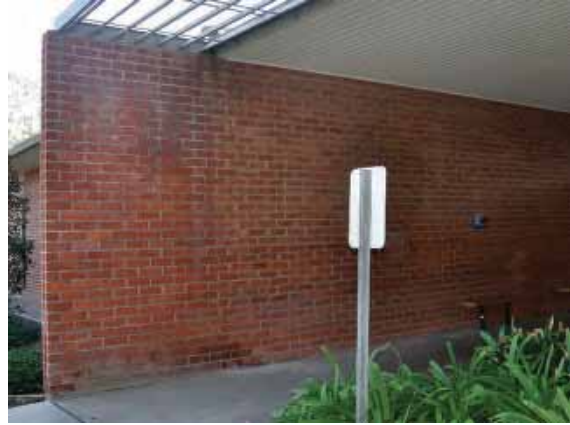
Figure 130: Efflorescence and algal growth on the west side of the projecting west façade.
