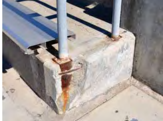
Figure 223: Heavy corrosion has resulted in oxide jacking and loss of a significant area of concrete on a corner at the east bleachers.
