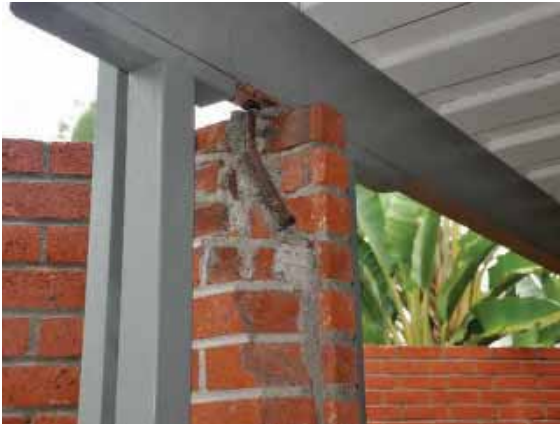
Figure 165: Oxide jacking causing the loss of brickwork on a brick wing wall at Building 35.
