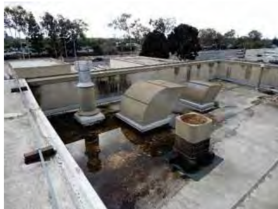
Figure 156: Water pooling within the dropped-level area on Building 2.
