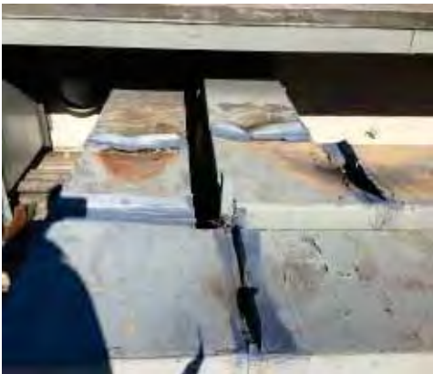
Damaged Ductwork from RTU within building 37
