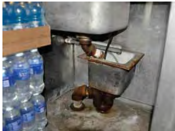
Figure 248: Rusted fixtures in the concessions room, Field House, Building 110.
