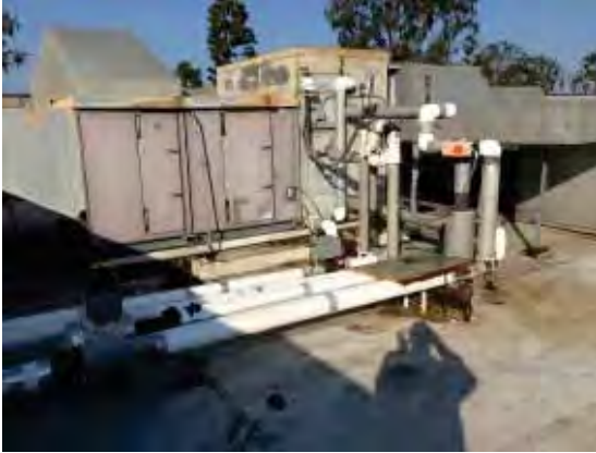
Multizone AHU on roof
