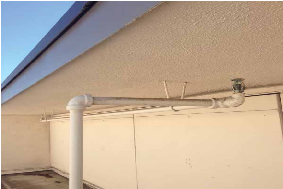
Photograph 9-View of the suspect exterior stucco, roof area
