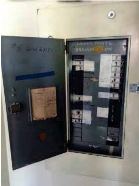
Existing unlabeled panel that should be replaced
