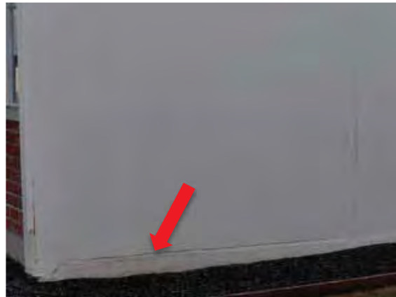
Figure 105: Crack/separation from the foundation slab at the base of the west façade of Building 9 and corrosion at corner.
