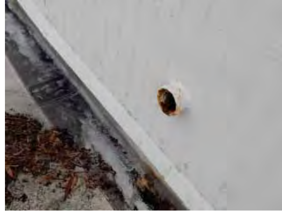
Figure 149: Rusted end of downpipe feeding water to flat roof to the south of the auditorium (Bldg. 2).
