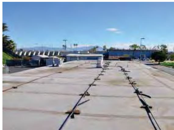
Figure 238: Corroded conduit (left) and remaining detached sheathing (center and right conduits) on the roof of the Field House facing east.
