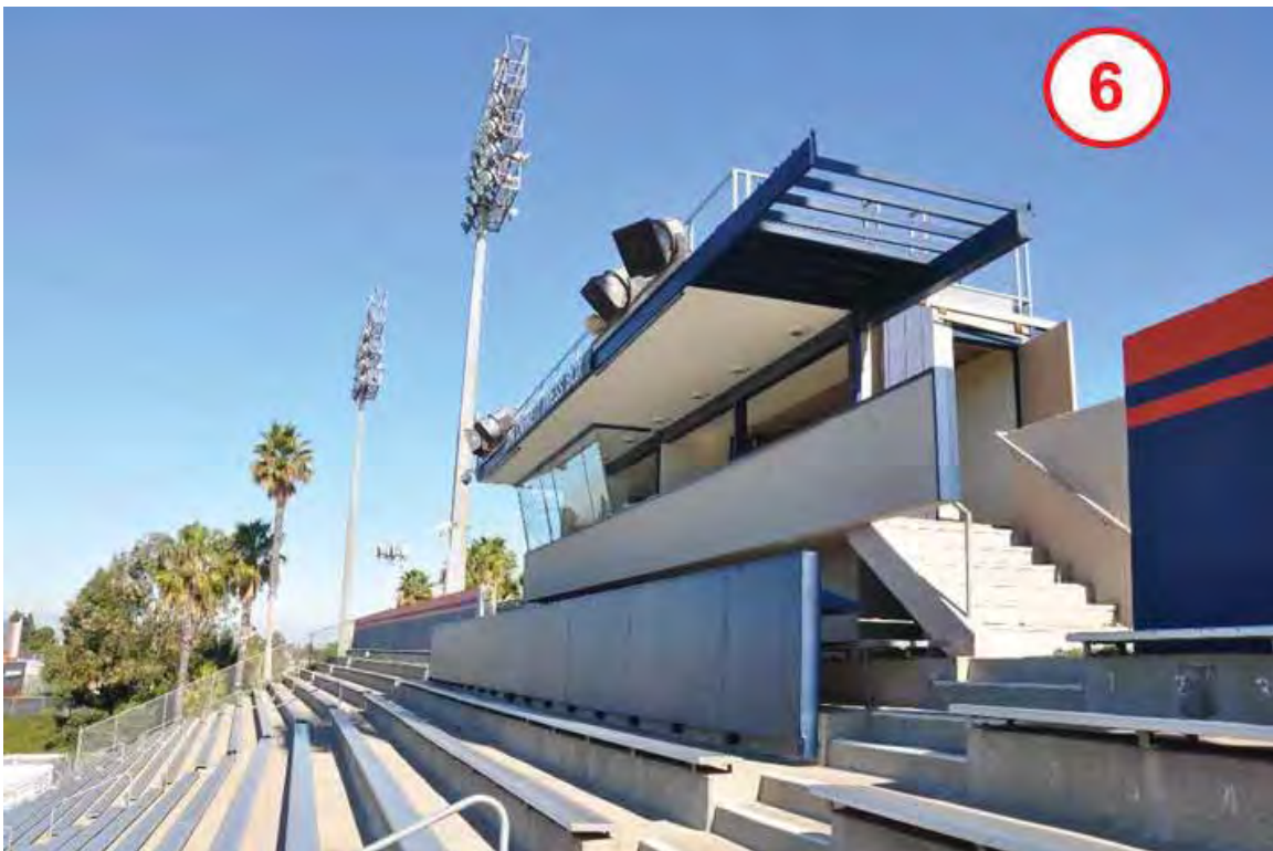
Figure 1D-36: Contemporary image of the Stadium and Press Box (Bldg. 105) with character defining features identified by red callouts.
