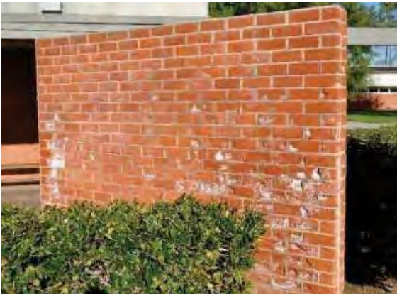
Figure 131: Wing wall on Building 12 showing efflorescence up to \frac{3}{4} of the height of the wall and spalling brickwork particularly at the right-hand side of the image.
