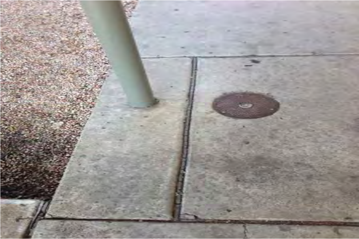
Photograph 6-View of exterior suspect expansion joint
