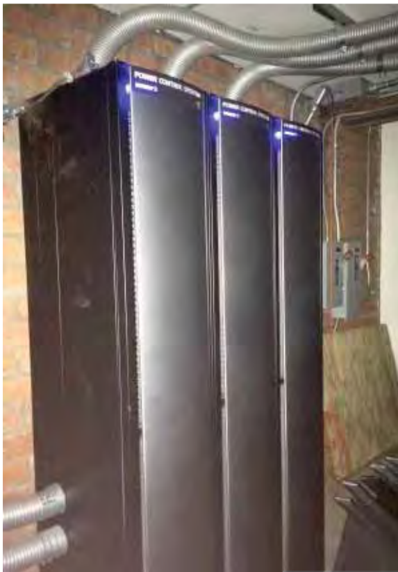
Existing dimmer racks
