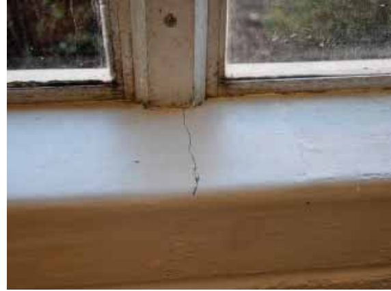
Figure 189: Cracking at steel mullions on internal painted concrete sill, Building 35.
