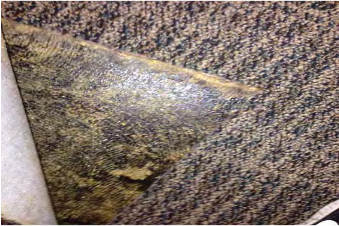
Photograph 8-View of the suspect floor mastic under the carpet
