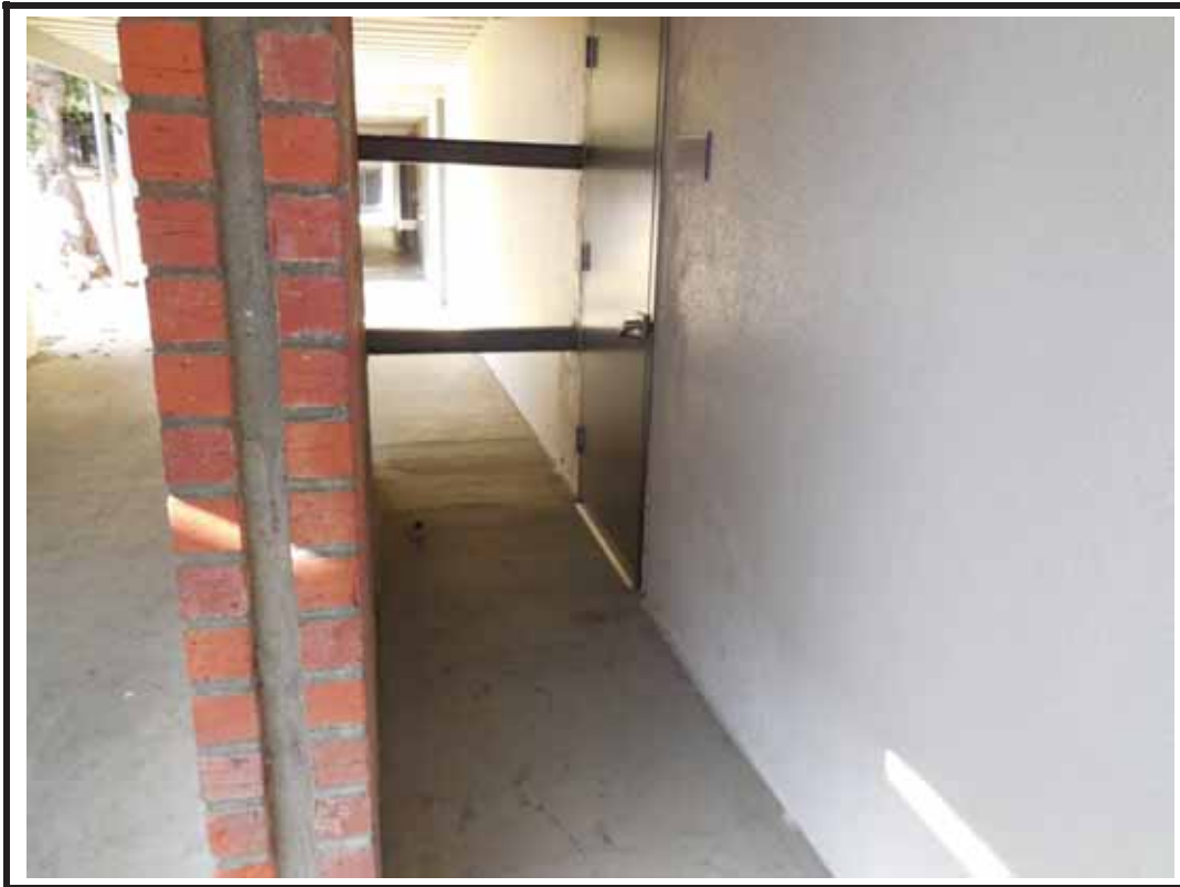
Photograph 9: Second exit door for Room 146 located in Building 36 impeded by brick wall.
