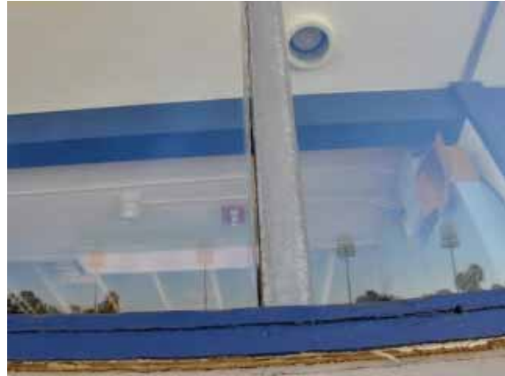
Figure 229: Gap between glazing and aluminum frame on east press box and deterioration of wooden sill.
