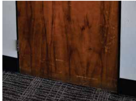
Figure 191: Wear and tear to original wood door in classroom, Building 35.
