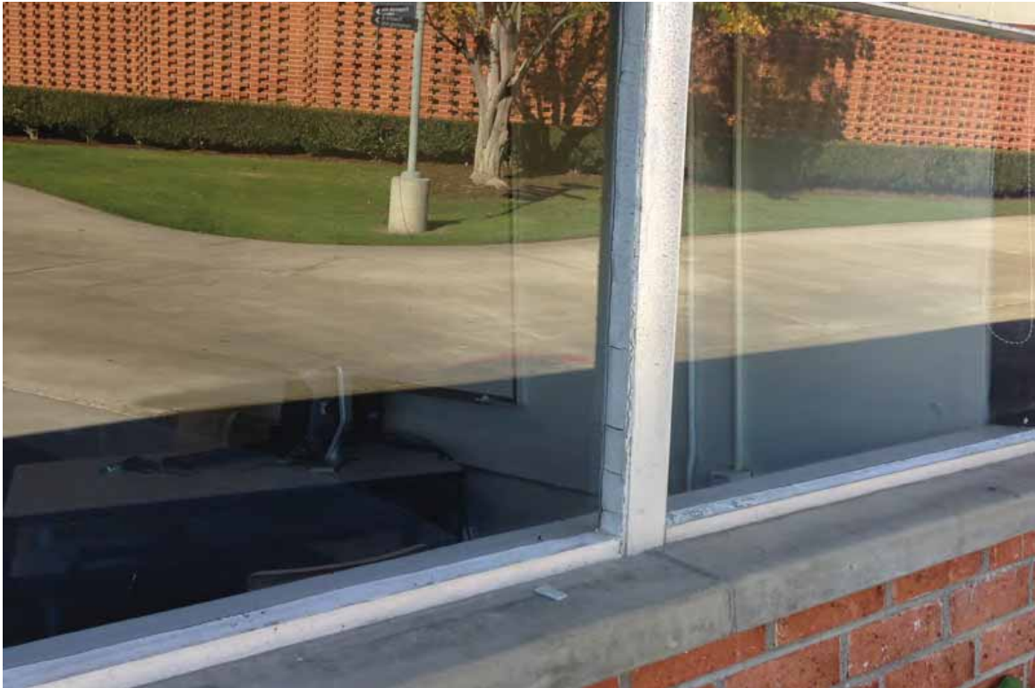
Photograph 4-View of the suspect exterior window putty and lead paint
