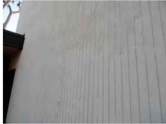
Figure 151: Patched finish on the east façade of Building 2.
