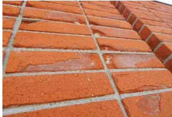
Figure 194: Surface spalls and hairline cracking on the brickwork on the east wall of the Swimming Pool complex.
