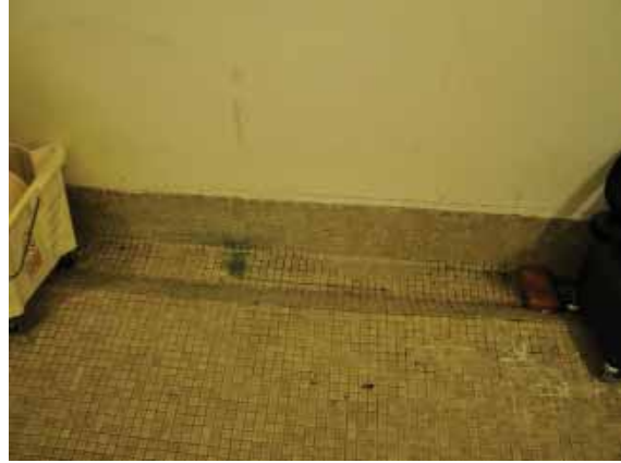
Figure 244: Signs of wear and tear on the wall and floor surfaces, Field House, Building 110.
