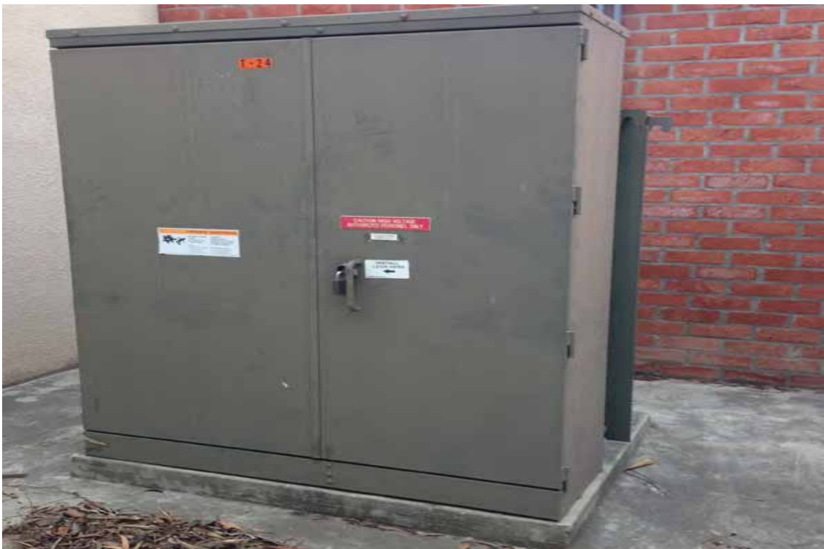
Photograph 16-View of the exterior transformer with suspect PCB materials
