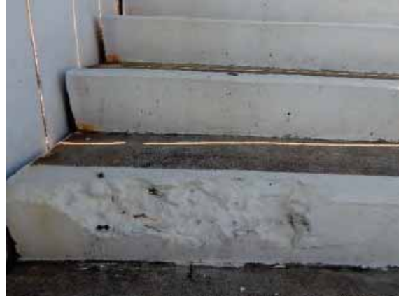
Figure 206: Missing material on the left-hand steps that has been painted over.
