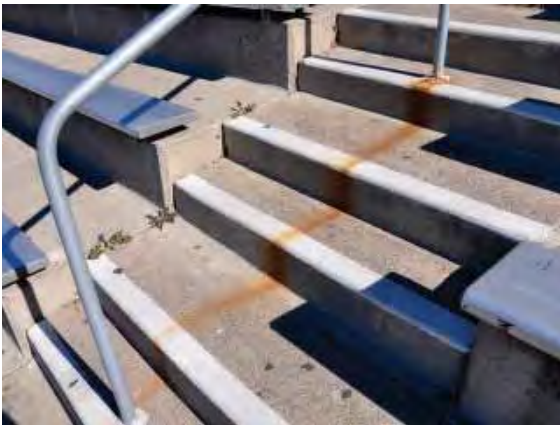
Figure 224: Corrosion of the base of a steel railing upright on the east bleachers has resulted in significant oxide staining on the steps below.
