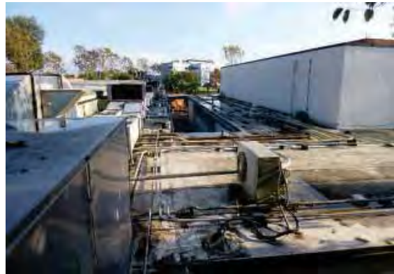
Figure 177: Water pooling and corroded pipes running across the roofs of Building 37 (right), 38 (center), and the walkway canopy neighboring Building 36 (left).
