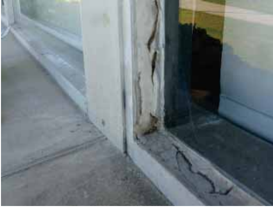
Figure 108: Cracked glazing putty on the north façade of Building 9.
