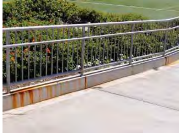
Figure 232: Significant levels of corrosion staining at the base of the railings on the ramp access to the stadium from the northwest corner.
