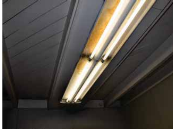
Figure 246: Water staining on light fixture in restroom indicating water ingress from roof, Field House, Building 110.
