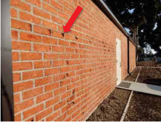
Figure 146: West façade of the Music Building showing loss of brick surface (Bldg. 4).
