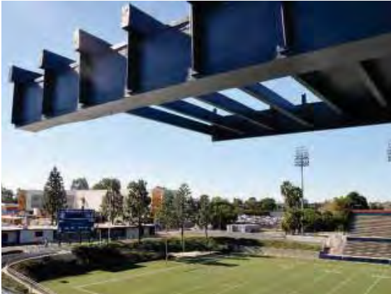
Figure 228: Roof structure overhanging to the south of the east press box showing some splits or checks in the wood beams.
