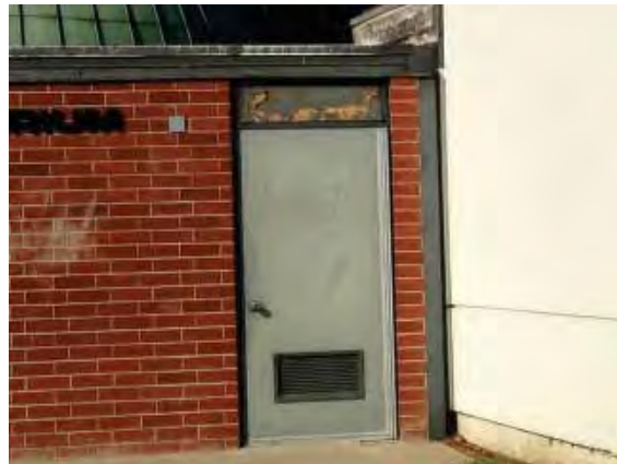
Figure 175: Graffiti and peeling paint from the transom on the east façade of Building 39.
