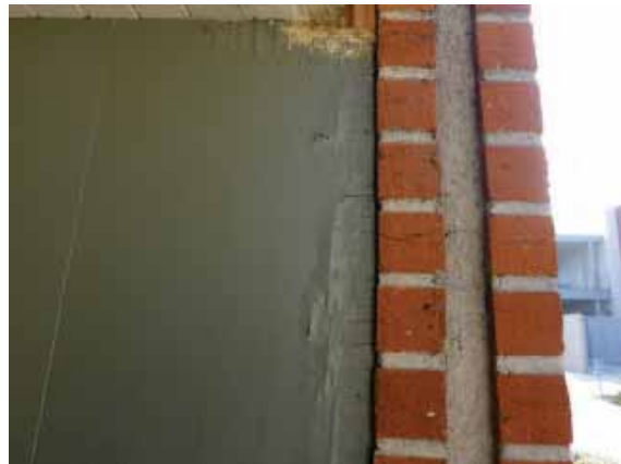
Figure 170: Water damage at edge of plywood paneling on Building 37 west façade.
