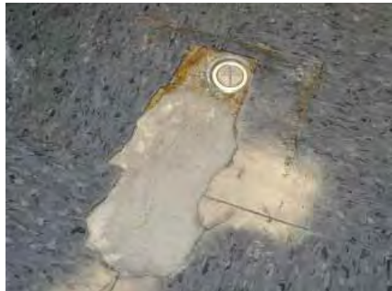
Figure 124: Damaged linoleum flooring in x-ray room South, Building 8.
