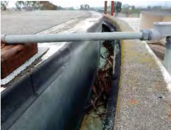
Figure 157: Plant detritus accumulation within the gutter on the theater auditorium (Bldg. 2).
