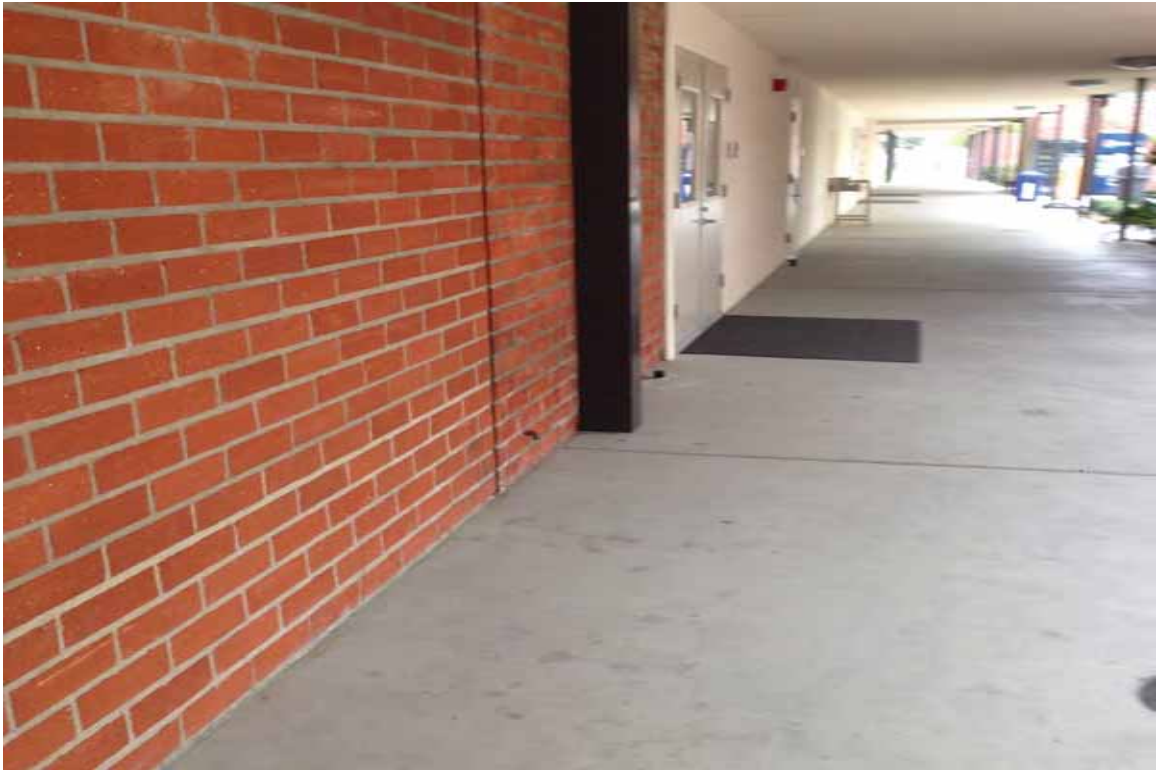
Photograph 12-General view of the suspect exterior building materials
