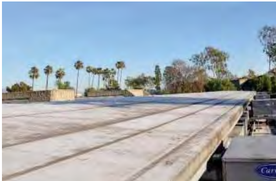
Figure 137: Light soiling and algal growth on the low-slope roof over Building 12.
