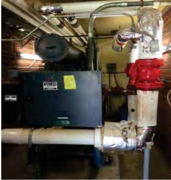
Trane water cooled chiller, showing pipe insulation
