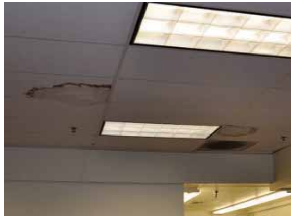
Figure 122: Areas of water staining on the acoustical tile in Room 102, Building 7.
