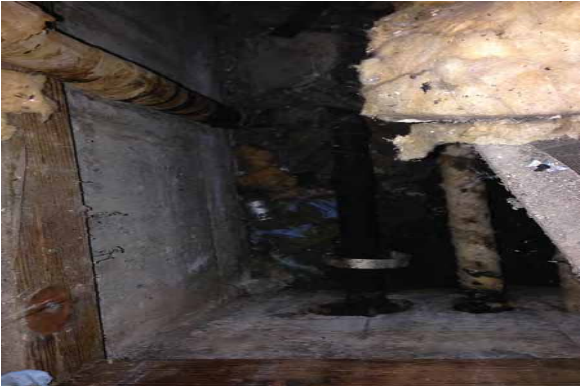
Photograph 8-View of pipe insulation & debris inside the mechanical room
