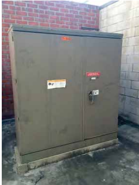
4160V Transformer T-24A
