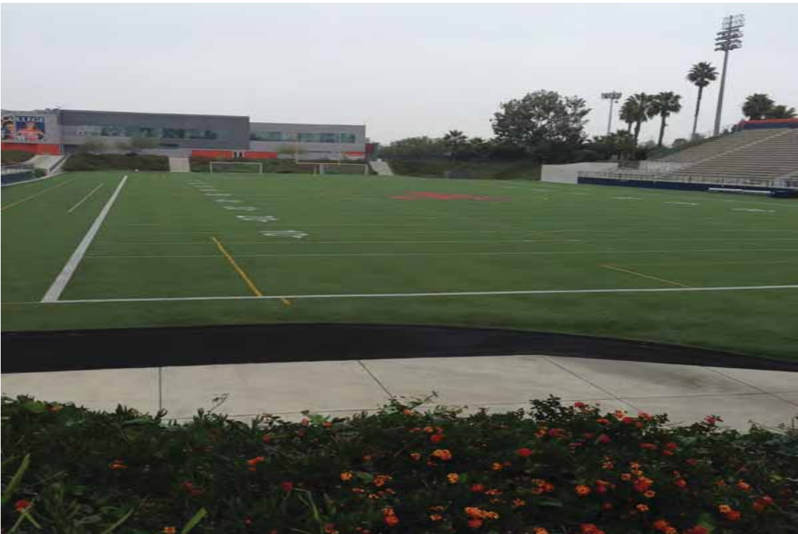
Photograph 8-General view of the Stadium with suspect lead paint
